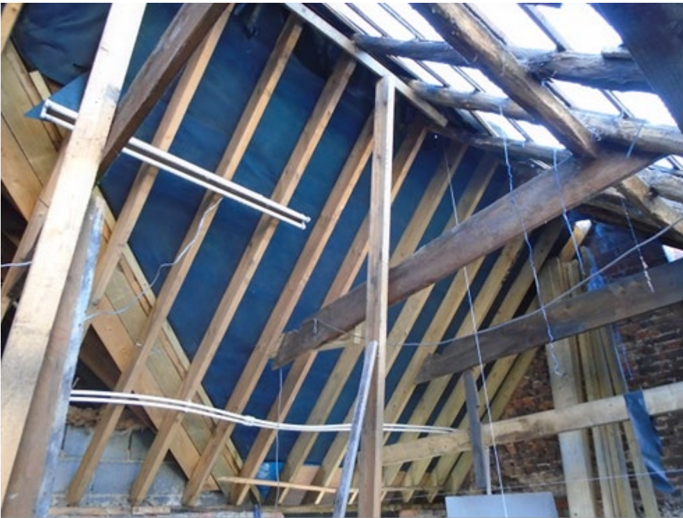
Figure 4: General view, facing south, of the largely replaced roof of the rear range (photograph Robert Howard)
