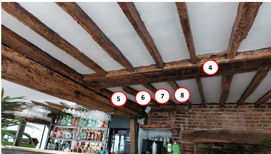
Figure 3c/d: Annotated photographs to help identify sample locations, first floor looking south-west (top) and looking south (bottom) [photographs Robert Howard]
