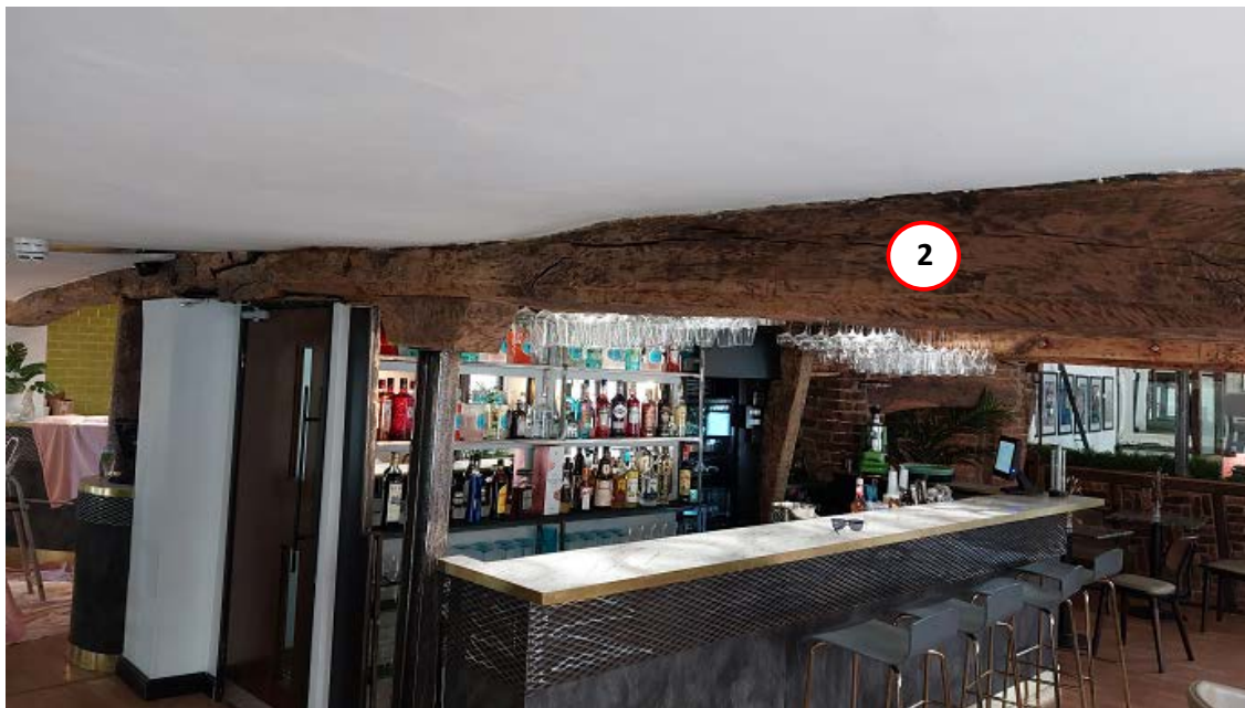
Figure 3a/b: Annotated photographs to help identify sample locations, first floor looking south-east (top) and looking south-west (bottom) [photographs Robert Howard]
