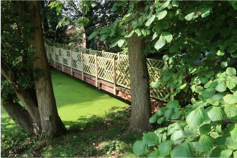
Figure 66: Ornamental footbridge [50] crossing the Mill Head in the gardens of Tonedale House, September 2021 [Johanna Roethe © Historic England]
