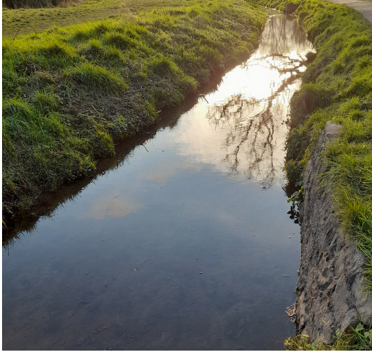
Figure 12: Leat [10], which leads to the Waterfall Weir, looking south-west away from the weir, January 2022 [Nicky Smith © Historic England]
