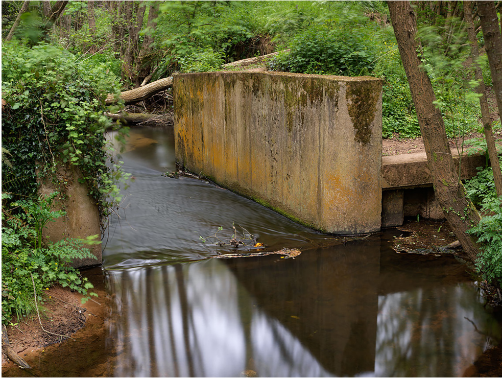
Figure 19: Concrete weir [8] built as part of flood alleviation work in the 1990s, looking north-east, April 2022 [James O. Davies © Historic England Archive, DP347750]
