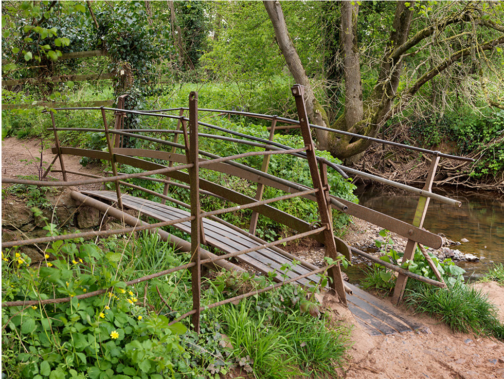
Figure 61: Blacksmith bridge [2] at Oaken Ground, bearing the date 1831 (not visible in this image), viewed from the south-east [James O. Davies © Historic England Archive, DP347762]
