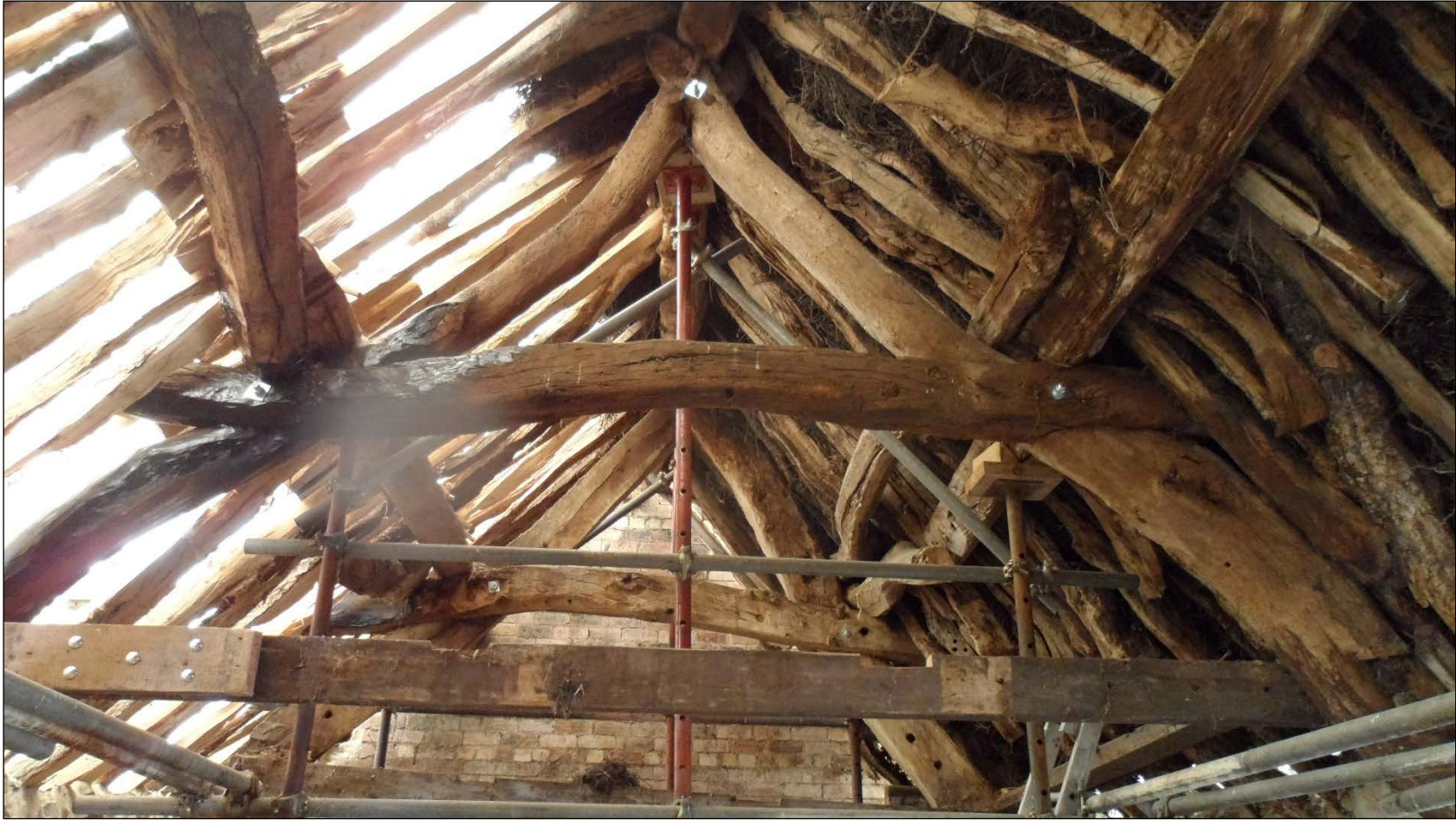
Figure 3: Photograph of the roof, with truss 2 in the foreground, photograph taken from the south-east (Alison Arnold)
