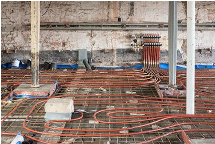
Figure 4: Underfloor heating on ground floor © Steve Baker, Historic England, March 2021
