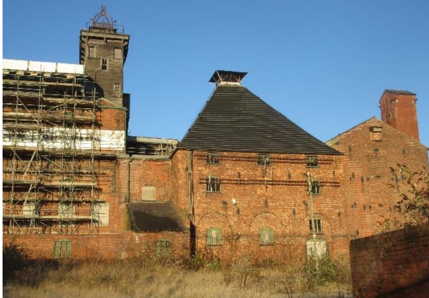
Figure 7: A view of the scaffolded Mill and tower, left, and boarded up Kiln, right © Historic England, December 2016
