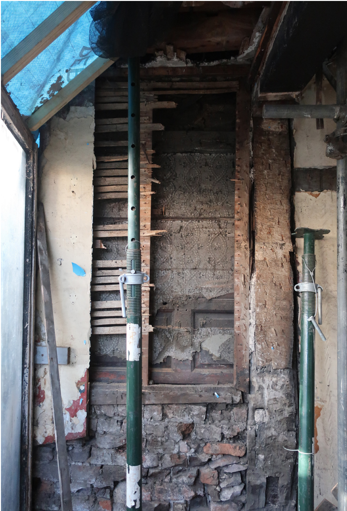
Figure 54: Timber panelling, possibly window shutters, used as part of the underbuilding of the jetty of the front range, now forming the partition between Nos 39 and 41, looking east. [Rebecca Lane © Historic England]
