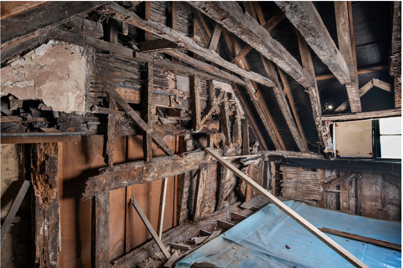
Figure 55: Raised roof over the western bay of the front range (No. 41) showing the later timbers inserted around the original gable-end framework, looking north-west. [James O. Davies © HEA DP435500]
