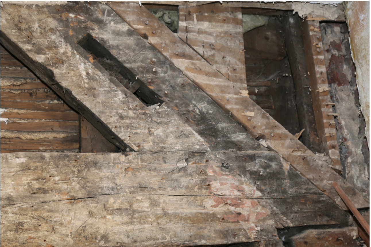
Figure 21: The central frame, showing the junction of the tie beam and principal rafter at the northern end, with a redundant mortice for a wind brace, looking west.[© Andrea Kirkham. Reproduced with permission]
