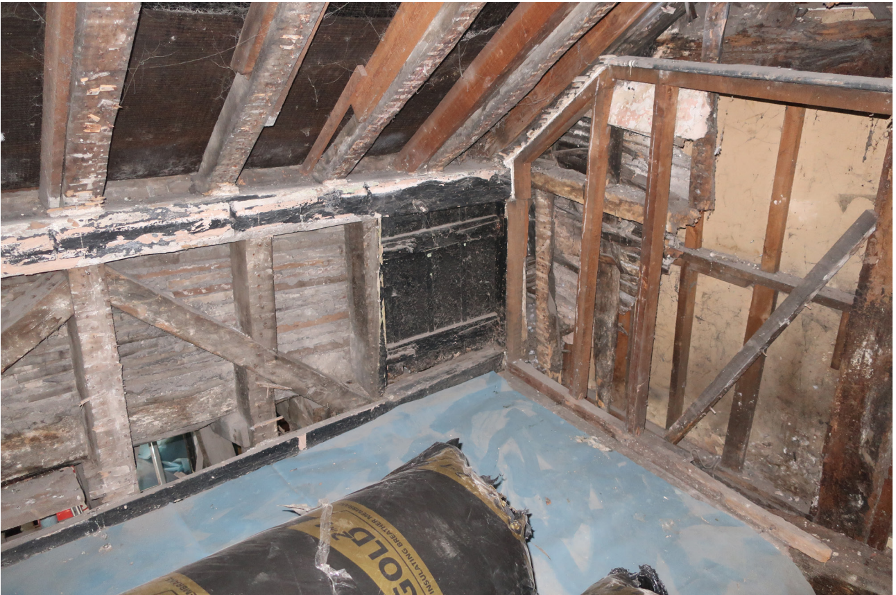
Figure 56: Raised wall line of the south elevation of the west bay of the front range (No. 41) showing the use of later timbers, and the reuse of the original wall plate at a higher level, looking south-west. [Rebecca Lane © Historic England]
