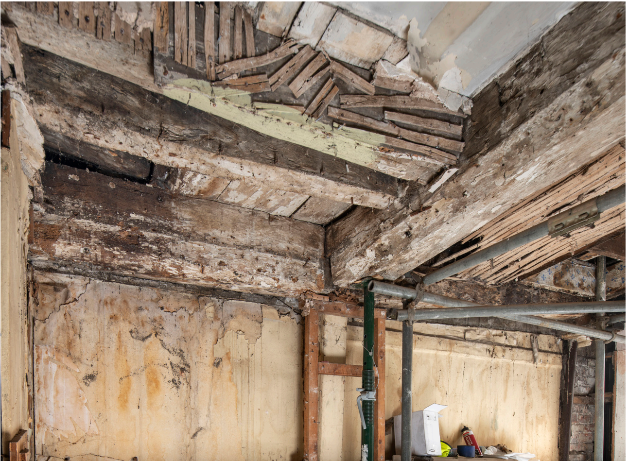
Figure 33: The main longitudinal beam in the western bay (No 41), where it meets the western frame (Frame C), showing simple chamfer moulding and straight-cut chamfer stop, looking north-west. [James O. Davies © HEA DP435518]
