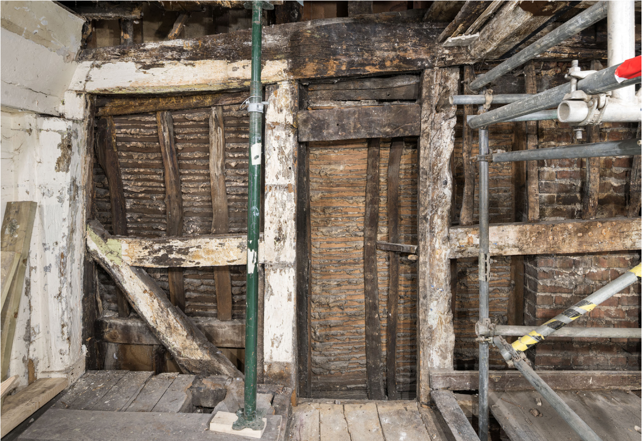
Figure 24: The southern section of the western frame (Frame C), showing the original doorway opening at first-floor level, looking west. [Steve Baker © HEA DP325698]
