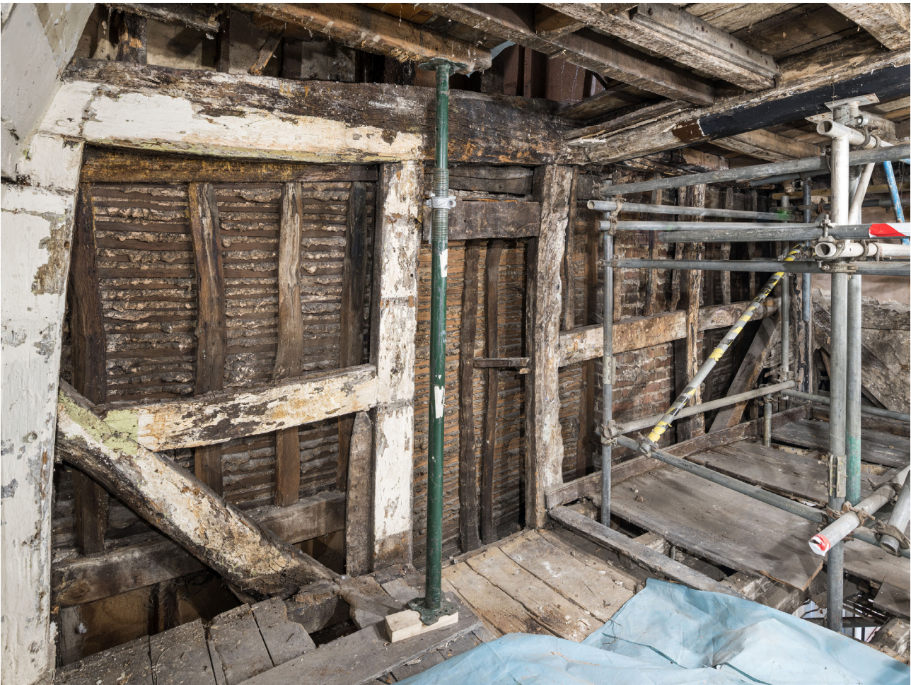
Figure 23: The western frame (Frame C) showing the surviving original framework at first-floor level, looking north-west. [Steve Baker © HEA DP325697]
