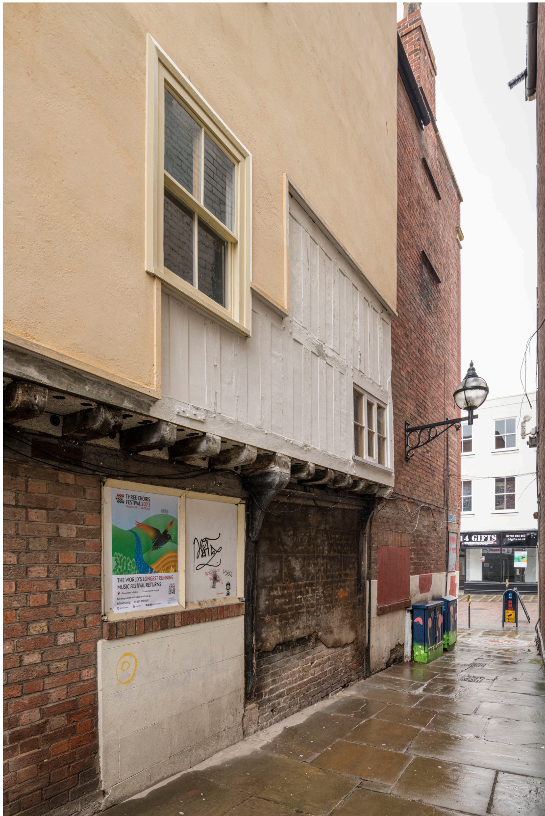
Figure 59: East elevation of the rear range of No. 39 at ground-floor level showing brick infill around the original timber posts, looking north. [Steve Baker © HEA DP464261]
