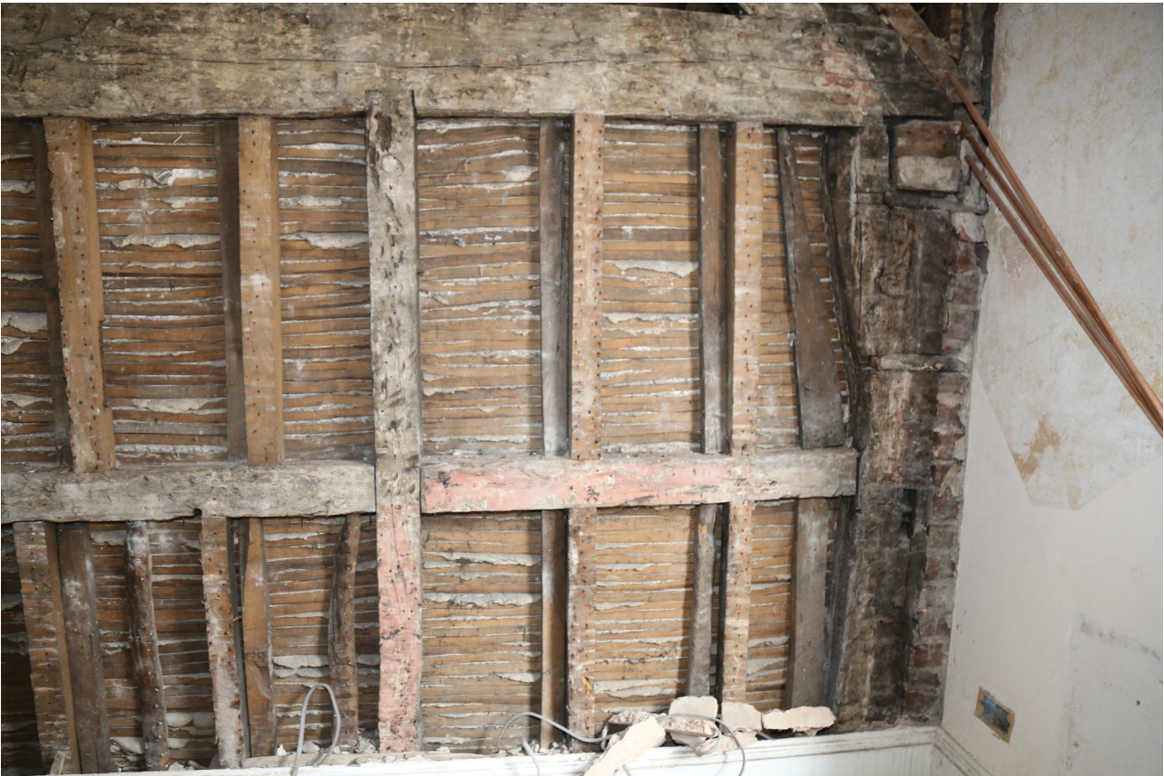
Figure 52: The north end of the central frame of the front range (Frame B), showing later framing lapped onto the original tie beam, looking west. [© Andrea Kirkham. Reproduced with permission]
