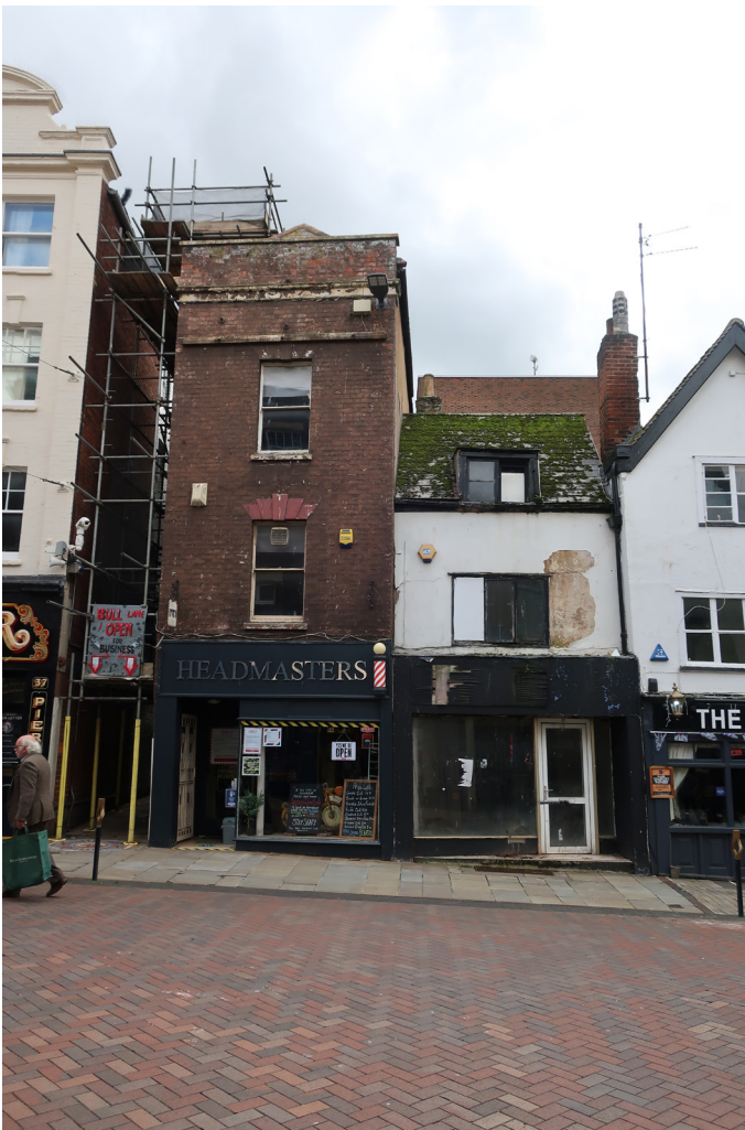
Figure 58: North elevation of Nos 39-41, prior to the recent restoration work, showing the eastern bay of the front range (No. 39) as rebuilt sometime between 1824 and 1834, looking south. [Rebecca Lane © Historic England]
