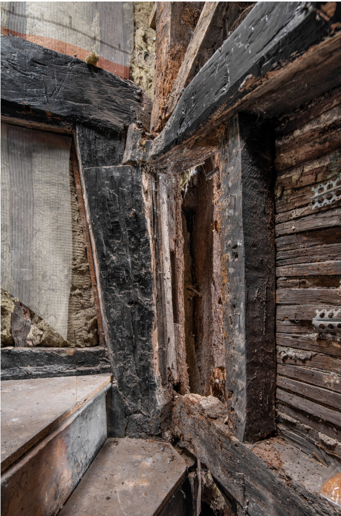
Figure 31: The south post of the central frame, showing redundant mortice for an up-brace, with later framing of the south elevation now projecting from it, looking south-east. [James O. Davies © HEA DP435492]
