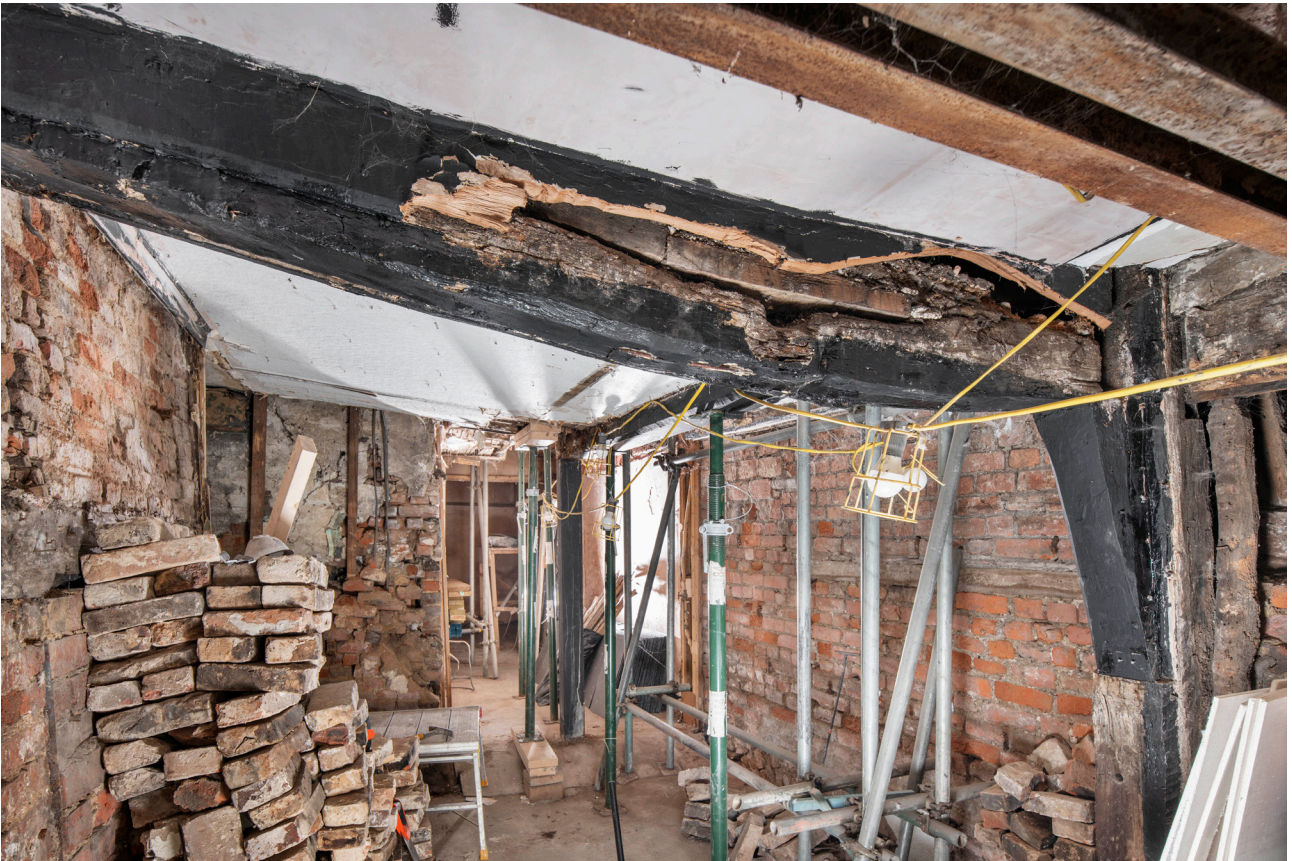
Figure 60: Rear range of No. 41, showing the later timber beam (now supported on acroprops) inserted to allow the removal of the ground-floor timber framing of the west elevation, running off the south girding beam of the front range, looking south-west. [James O. Davies © HEA DP435512]
