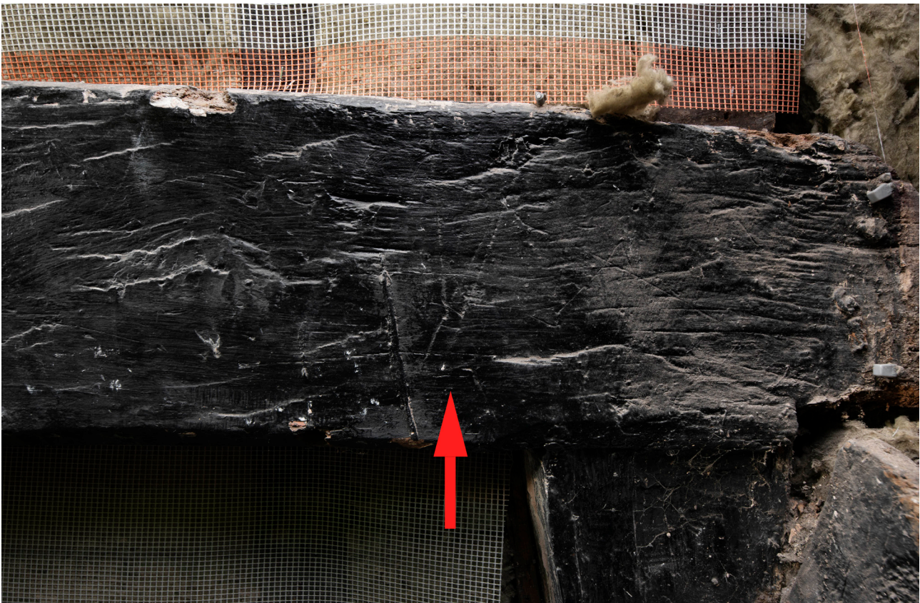
Figure 17: Carpenter's mark on the western side of the central frame of the front range (Frame B), looking east. [James O. Davies © HEA DP435493]
