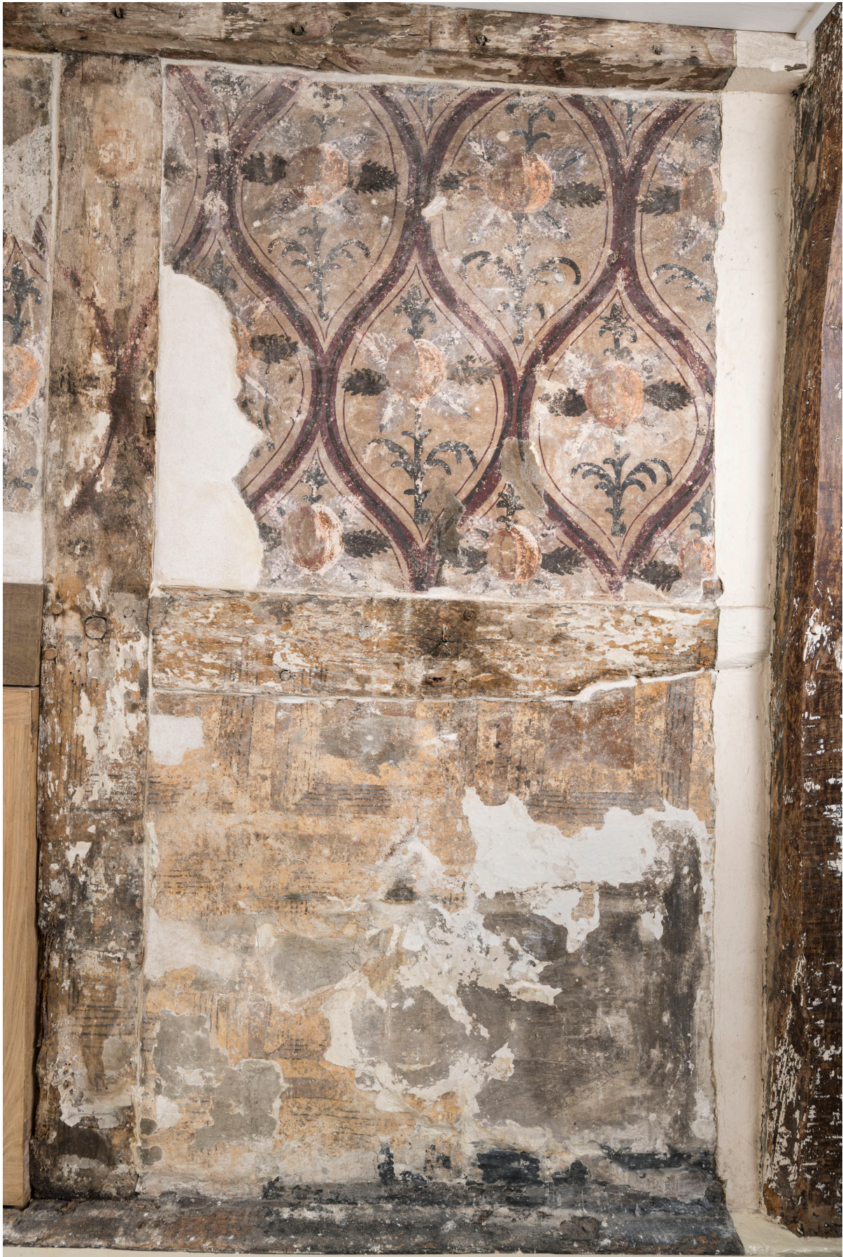
Figure 43: Painted wall scheme on the east elevation of the rear range, showing the imitation panelling on the bottom half and the lattice work above. [Steve Baker © HEA DP464281]
