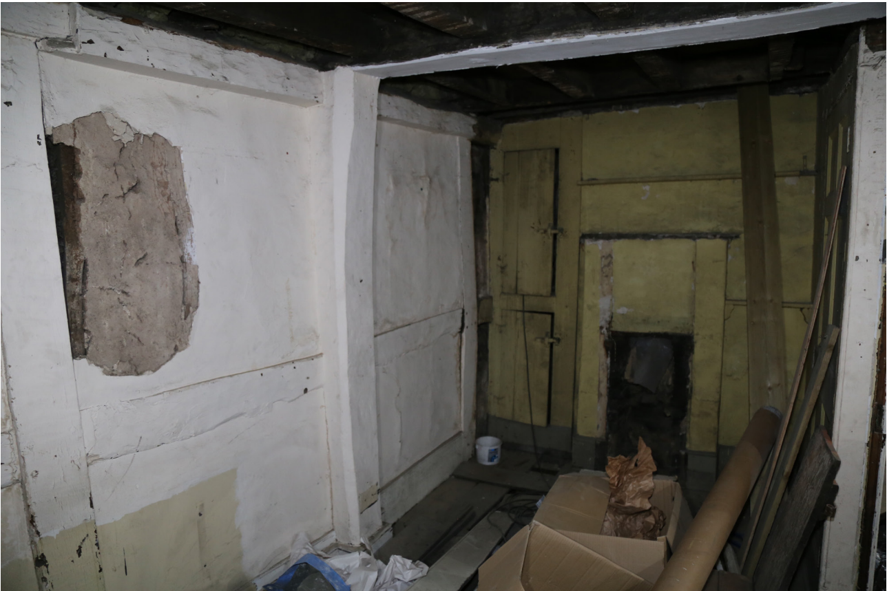
Figure 36: The west post of the central frame (Frame E) of the rear range of No. 39, also showing the box framing of the west wall of the range, and the later inserted chimney stack in the northern bay of the range, looking north-west. [© Andrea Kirkham. Reproduced with permission]
