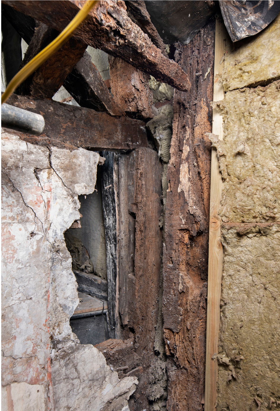
Figure 35: The south post of the central frame of the front range (Frame B), and the west post of the north frame of the rear range of No. 39 (Frame D), showing the later post butting up against the earlier one, looking north-east. [James O. Davies © HEA DP435485]
