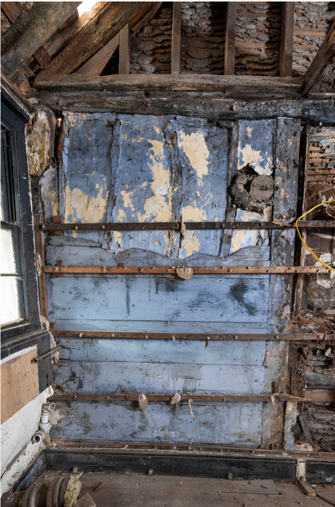
Figure 49: The south end of the west elevation of the rear range of No. 41 (Frame G), showing the original timber infill below the tie beam (partly hidden by later boarding) looking west. [James O. Davies © HEA DP435480]
