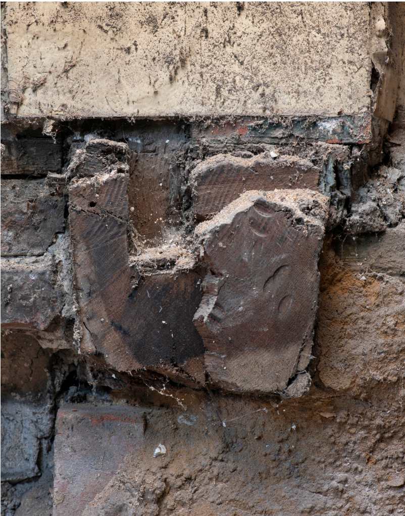
Figure 29: Sawn off end of the sill beam of the north elevation, visible from the western bay (now No. 41), looking east. [James O. Davies © HEA DP435523]
