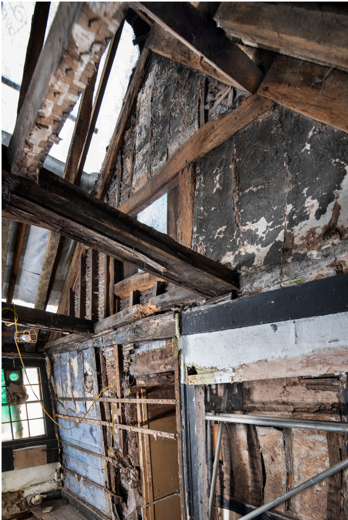
Figure 48: The gable end of the west elevation of the rear range of No. 41 (Frame G), looking south-west. [James O. Davies © HEA DP435488]
