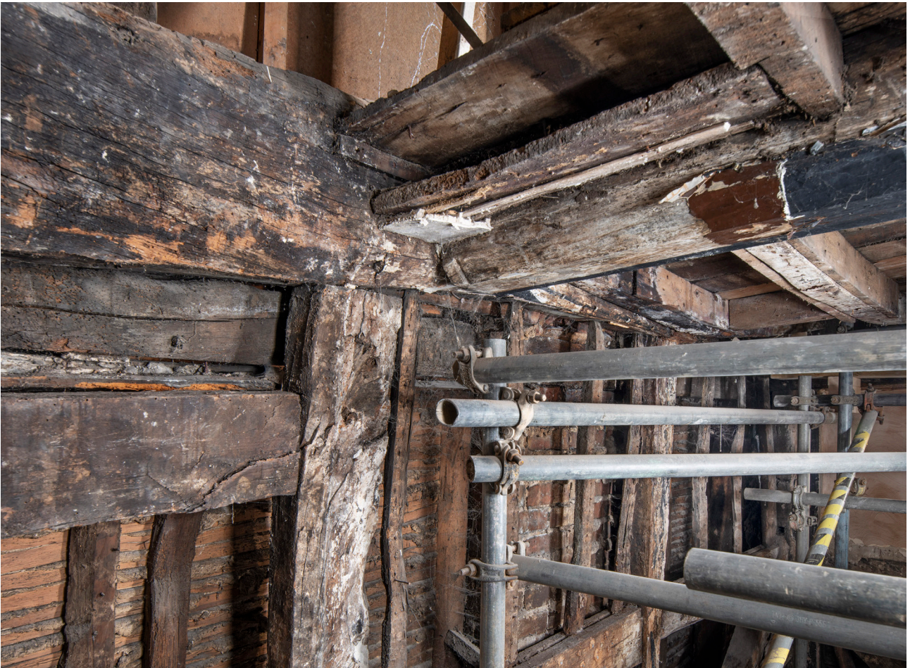
Figure 34: The ceiling arrangement at first-floor level in the western bay (No. 41), showing chamfer moulding to main beam with a stepped chamfer stop. [James O. Davies © HEA DP435495]
