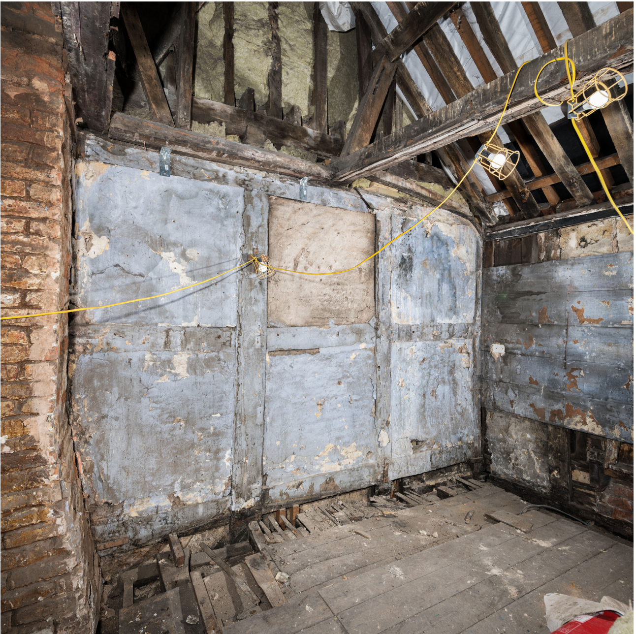
Figure 41: Framing of the west wall of the rear range of No. 39 (from within No. 41) showing box-frame form, looking south-east. [Steve Baker © HEA DP325694].
