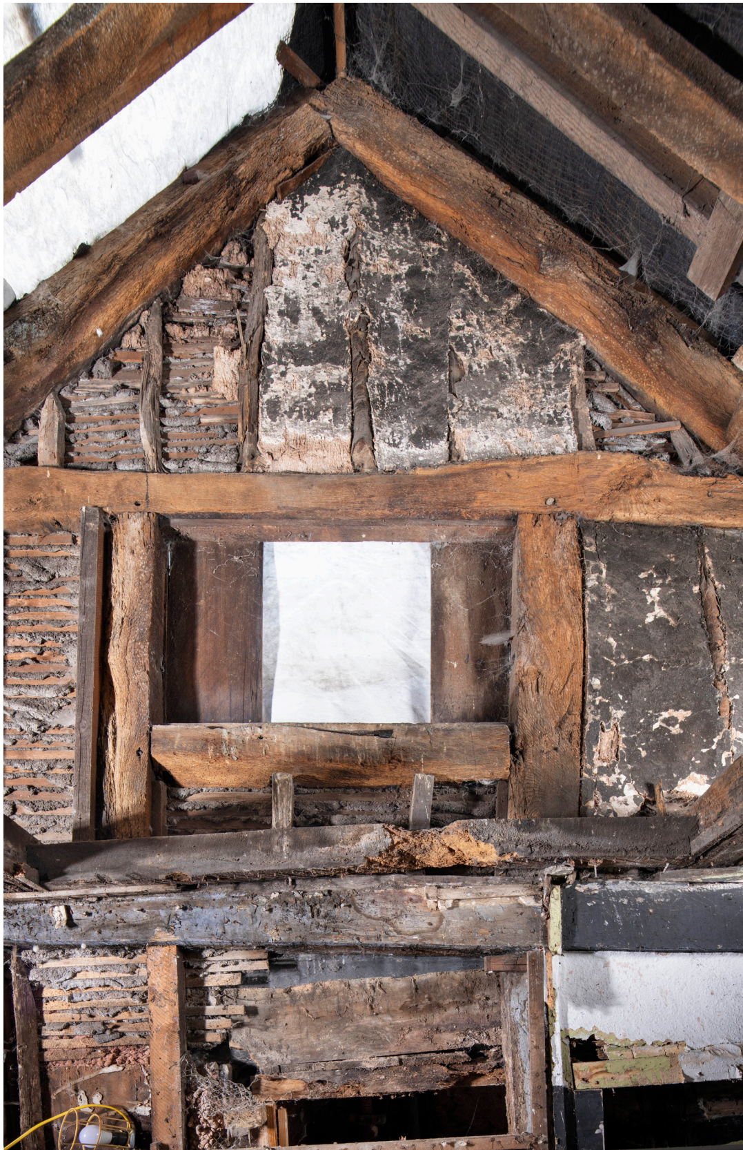
Figure 50: The gable end of the west elevation of the rear range of No. 41, showing the central window opening and original infill panels with staves to either side, looking west. [James O. Davies © HEA DP435482]
