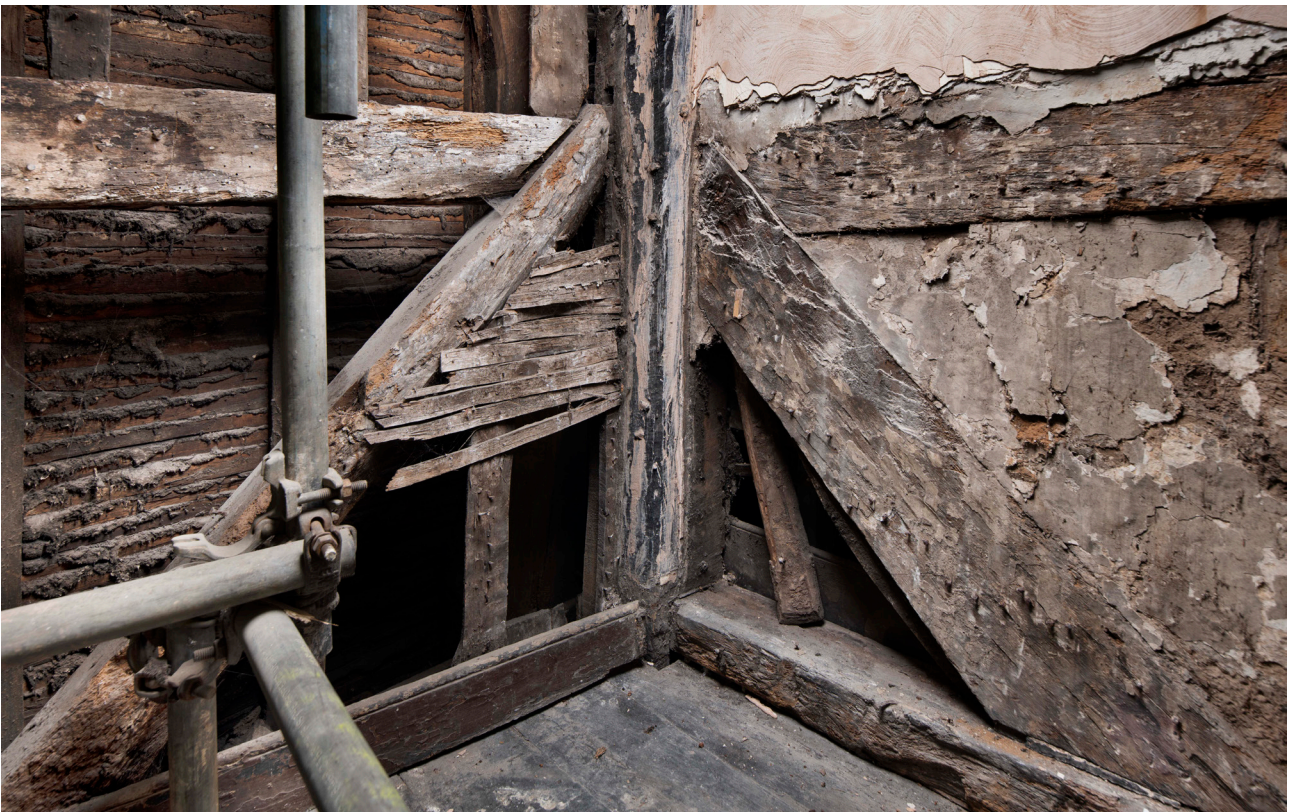
Figure 25: The corner brace at the north end of the western frame (Frame C), with the brace on the north elevation also shown, looking north-west. [James O. Davies © HEA DP435496]
