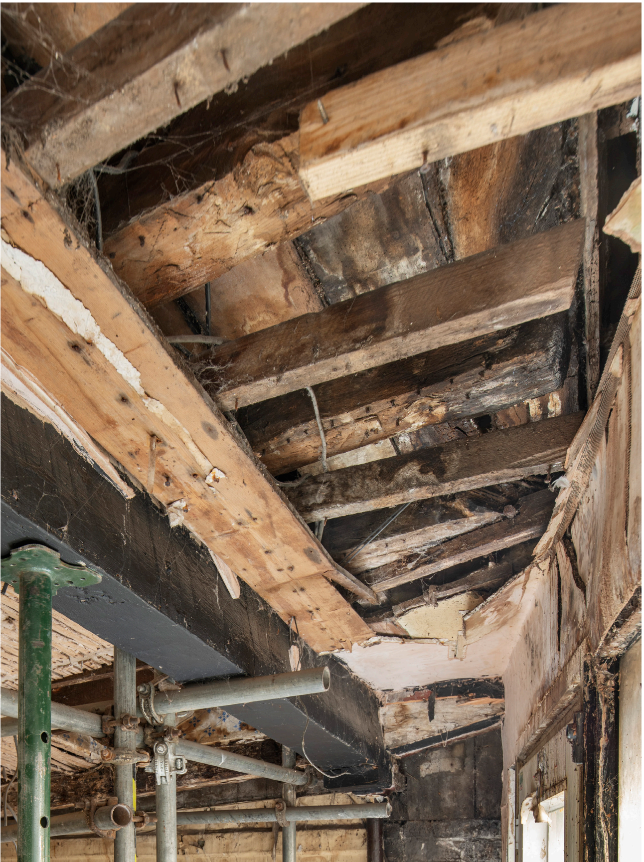
Figure 30: The jetty bressummer (painted black) and projecting joists, now within the front area of the western bay (No. 41), looking west. [James O. Davies © HEA DP435521]
