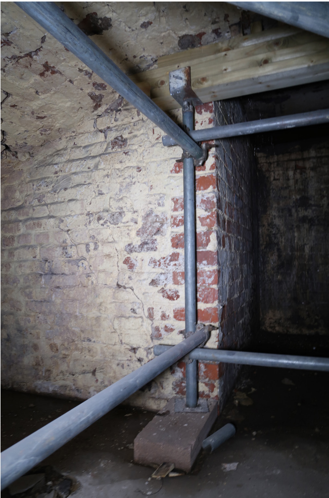
Figure 15: The cellar under No. 39, showing north wall with segmental-arch vaulted ceiling, looking north-west. [Abigail Lloyd © Historic England]
