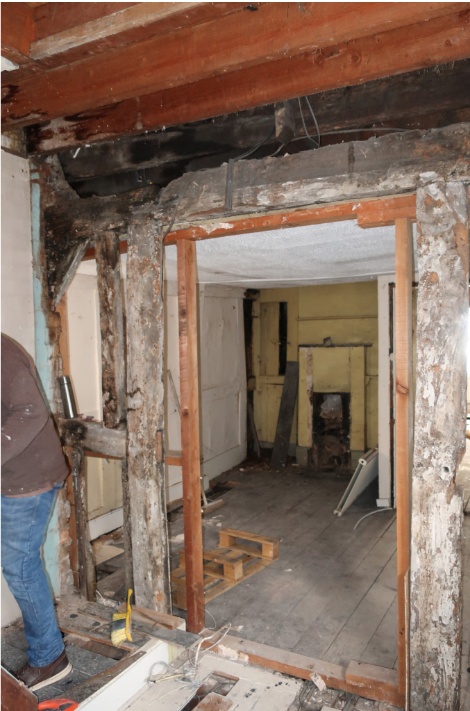
Figure 38: The southern frame of the rear range of No. 39, showing surviving framing at first-floor level, looking north-west. [Rebecca Lane © Historic England]
