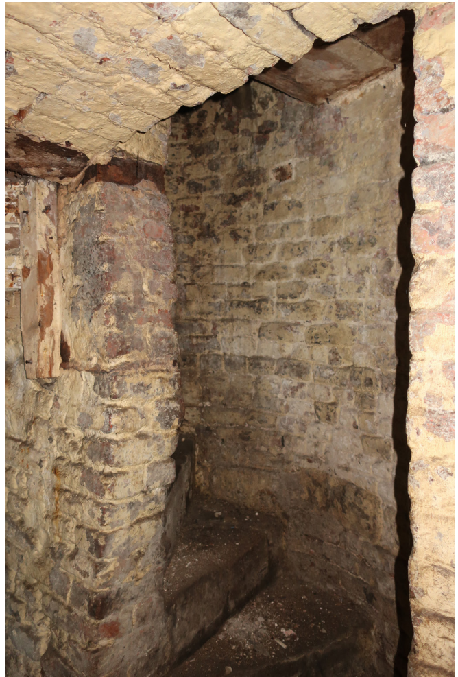
Figure 16: Brick stair rising from cellar to the rear of No. 39, looking south-east. [Rebecca Lane © Historic England]
