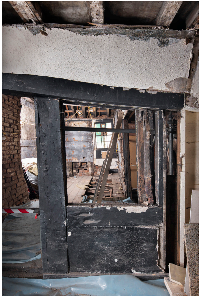
Figure 32: The later framing at the west end of the south elevation (No. 41), showing an original vertical stud reused in the elevation, looking south. [James O. Davies © HEA DP435491]
