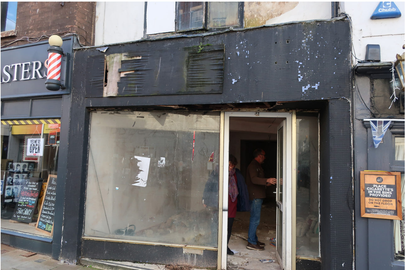
Figure 61: Shopfront inserted into the north elevation of No. 41 in the 20th century, looking south. [Rebecca Lane © Historic England]
