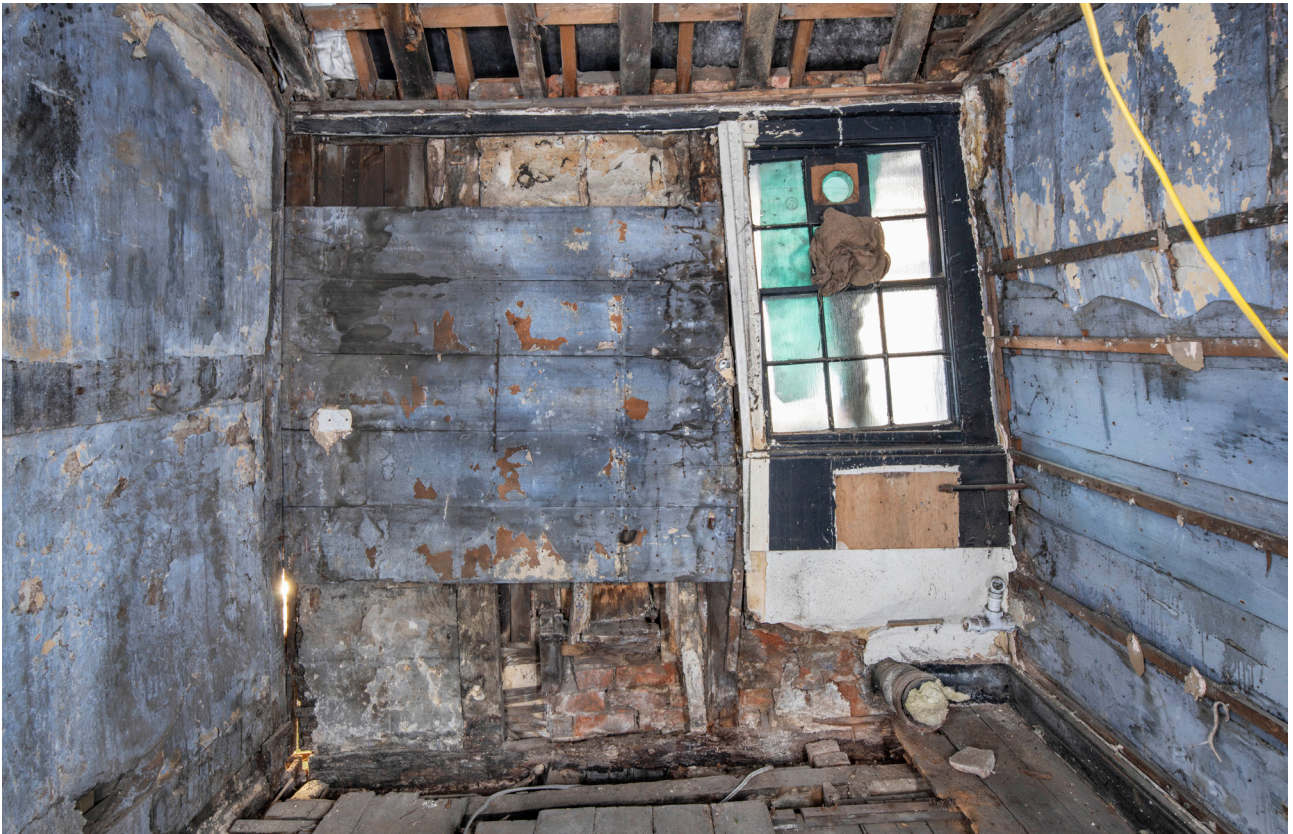
Figure 45: South elevation of the rear range of No. 41, showing framing and later timber boarding, looking south. [James O. Davies © HEA DP435478]
