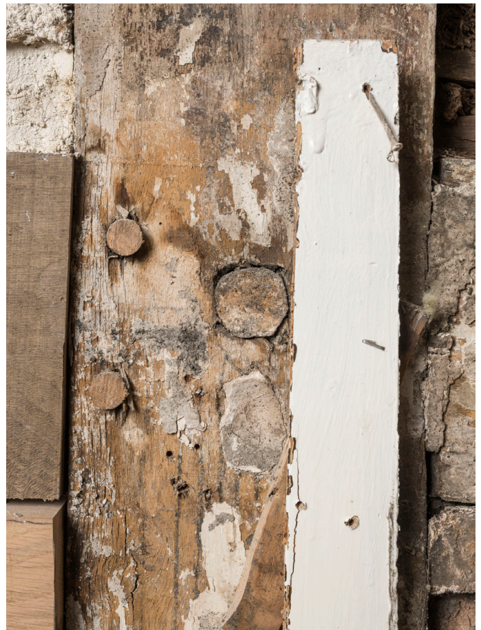
Figure 40: Face-peg on the timber frame of the east elevation of the rear range of No. 39, possibly to support original shelving, looking east. [Steve Baker © HEA DP464273]
