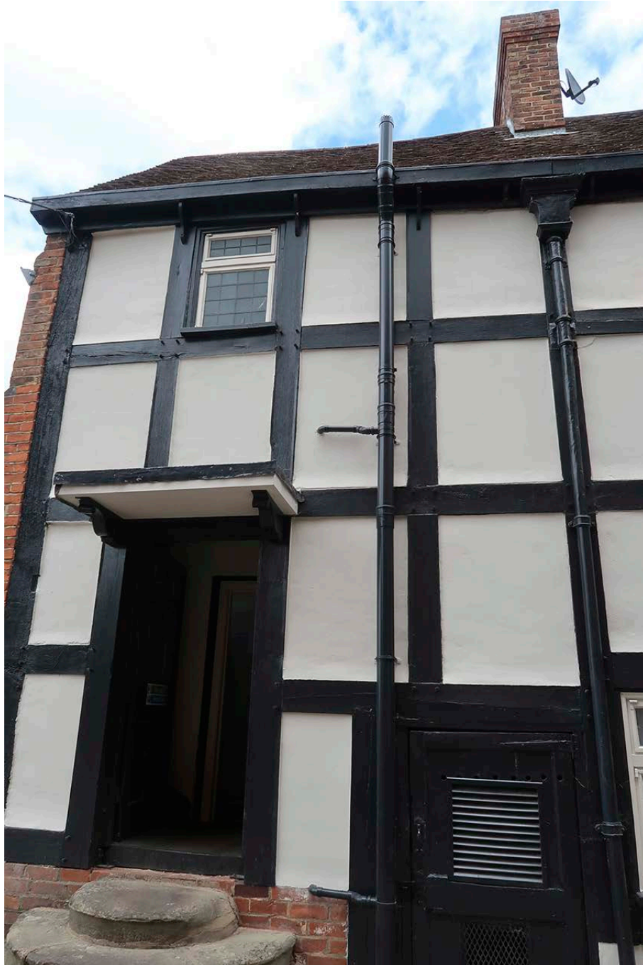
Figure 88: The west end of the north wing's south elevation. The later replacement of the timber framing masks the change in phase, which is marked by the downpipe with an early hopper. [Johanna Roethe © Historic England]
