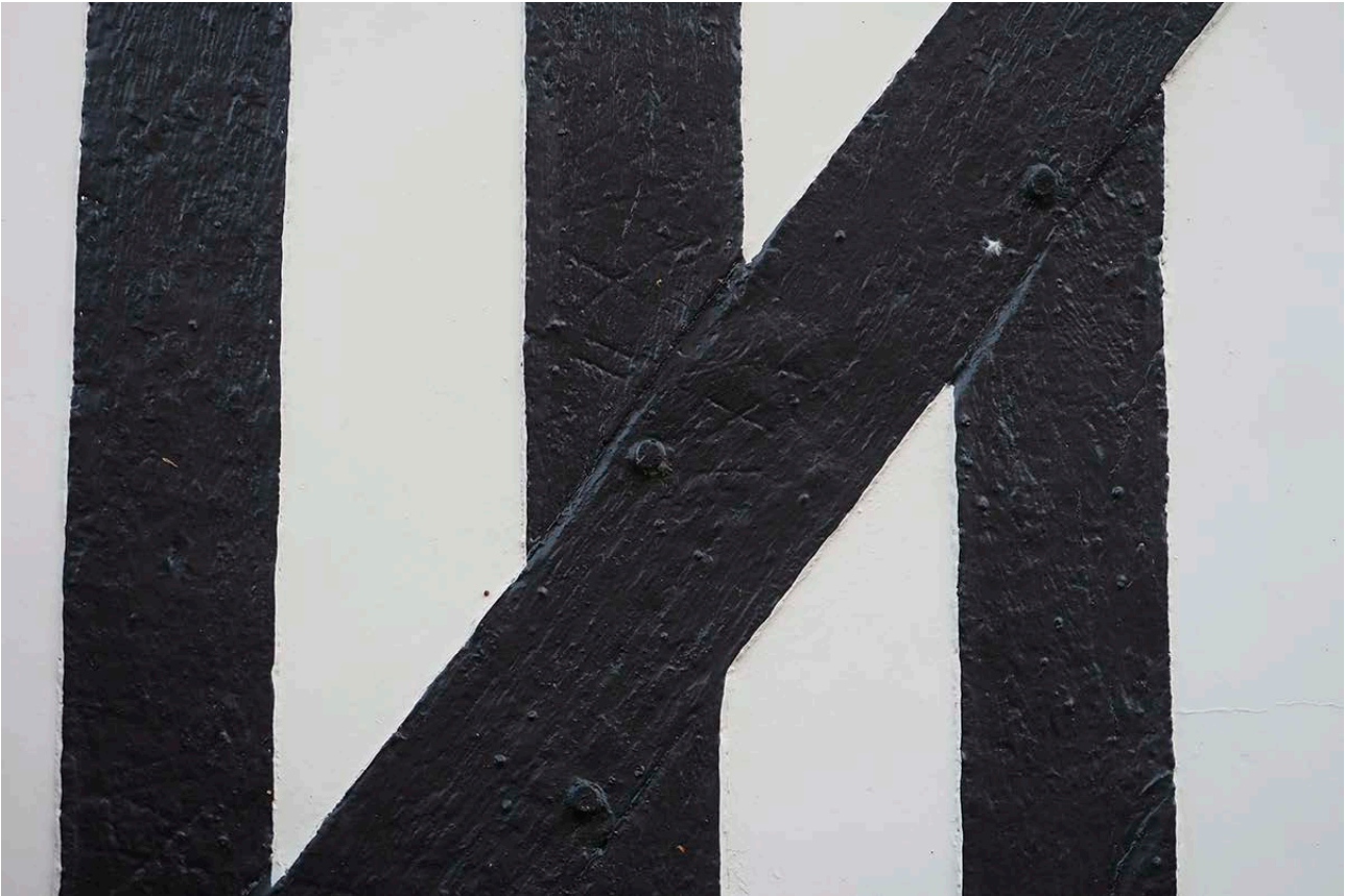
Figure 37: Detail of the framing in the eastern half of the north elevation, showing carpenter's marks with the number XII (for 12) on a stud and brace. [Abigail Lloyd © Historic England]
