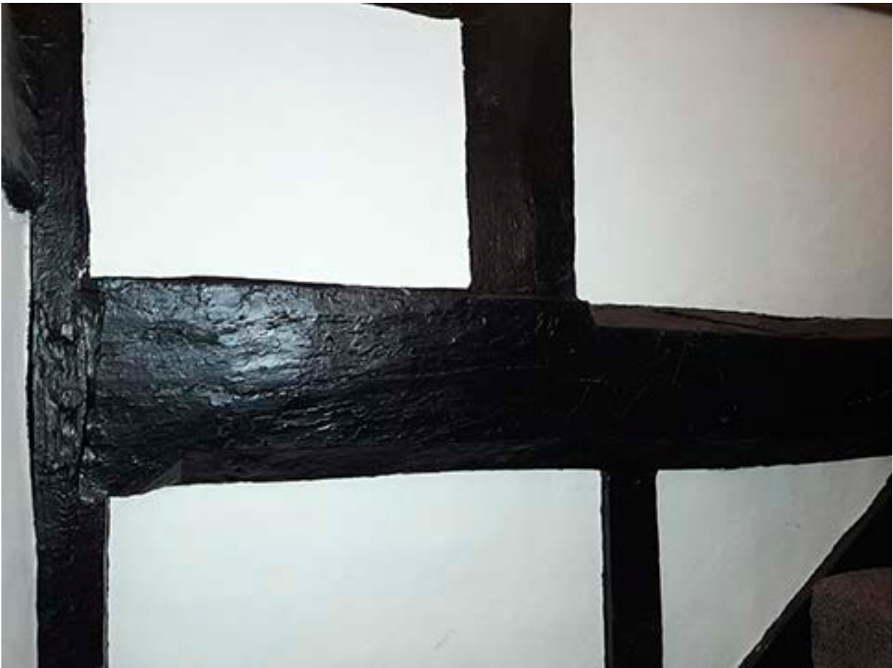
Figure 49: The chamfered girthing beam of the fourth truss from the west, just west of the stairwell. [Johanna Roethe © Historic England]
