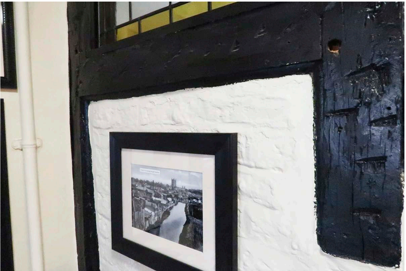
Figure 55: The moulded door frame at the east end of the stairwell's north wall, at ground-floor level, with later brick infill. [Johanna Roethe © Historic England]
