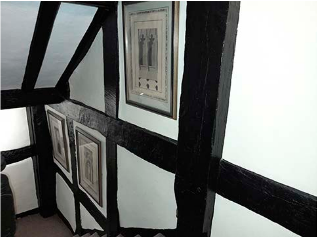
Figure 43: The south wall in the staircase looking down from the first-floor landing. [Johanna Roethe © Historic England]
