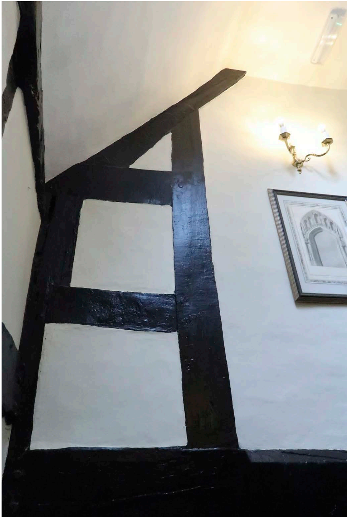
Figure 47: The south side of the fourth truss from the west. [Johanna Roethe © Historic England]
