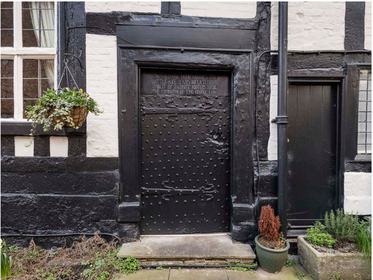
Figure 71: The main door in the north wing's north elevation. [Steven Baker © Historic England Archive, DP325762]
