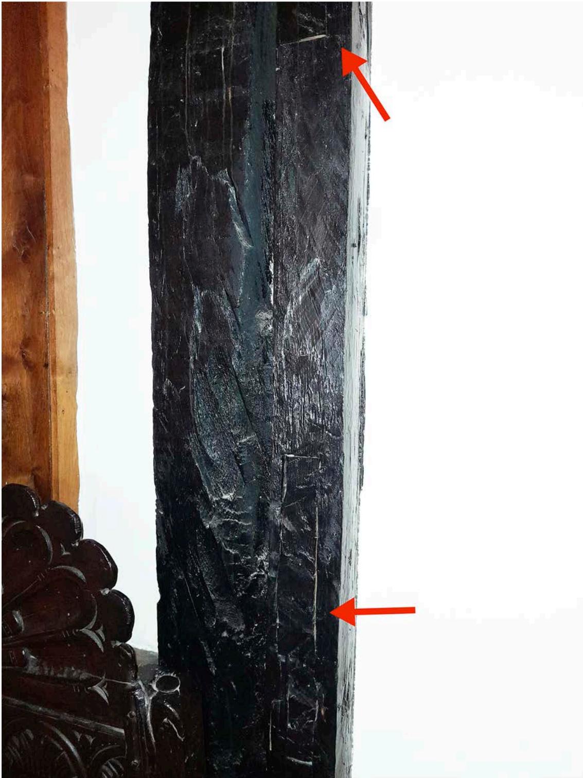
Figure 64: The mortices in the wall post just north of the stair enclosure's projecting partition at first-floor level. [Johanna Roethe © Historic England]
