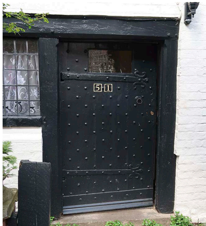
Figure 92: The door in the east elevation of the stable block. [Abigail Lloyd © Historic England]
