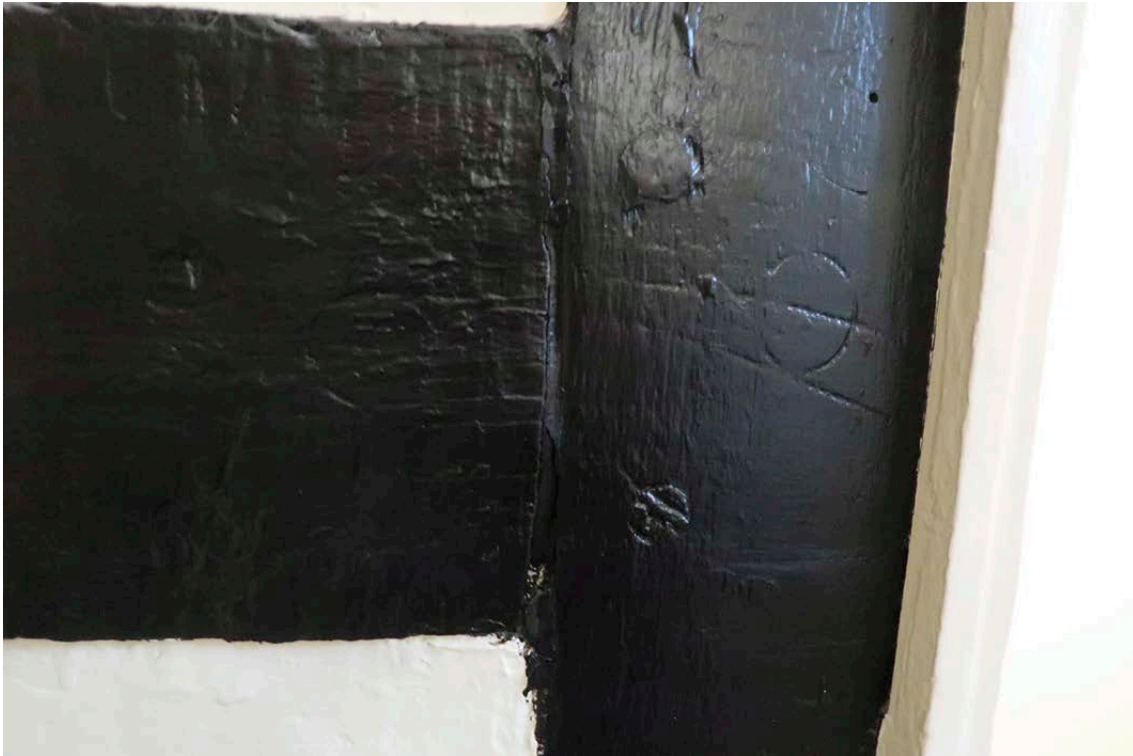
Figure 52: Carpenter's marks on the north end of the easternmost truss with the number 2 on both the mid-rail (left) and the strut (right). [Johanna Roethe © Historic England]
