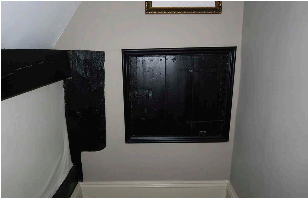
Figure 45: The south-west corner of the south wing at attic level. The south corner post of the westernmost frame is to the left and the chimneystack is to the right. [Johanna Roethe © Historic England]
