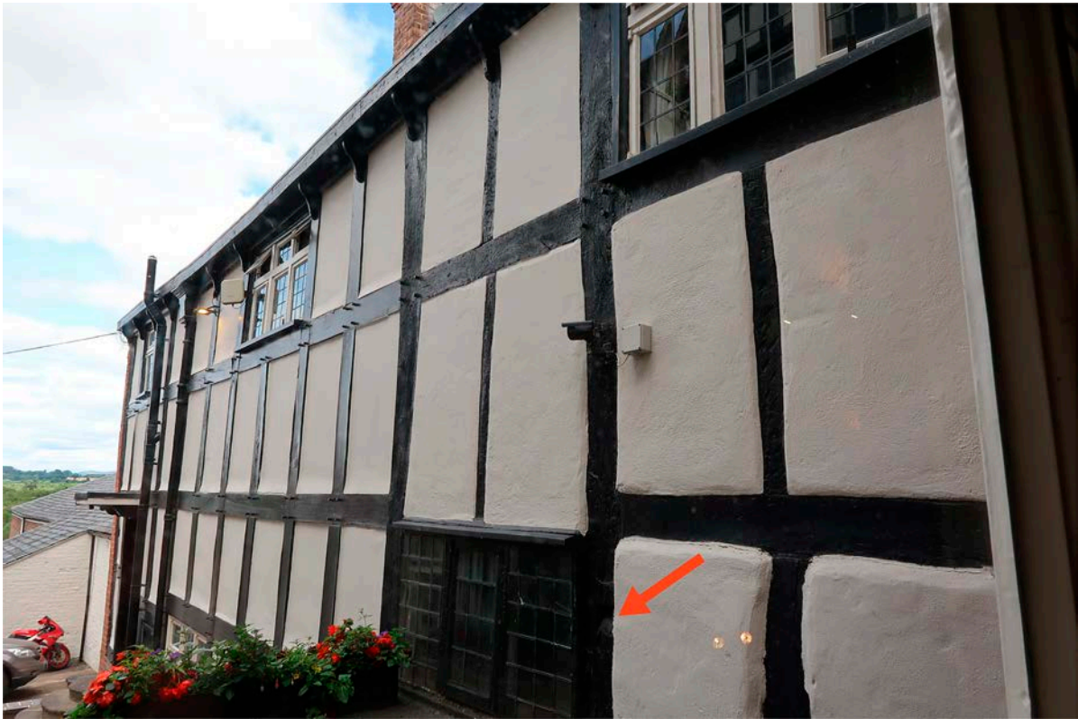
Figure 75: The south elevation of the north wing, seen from the stair west of the front range. The arrow indicates the location of the scotch. [Johanna Roethe © Historic England]
