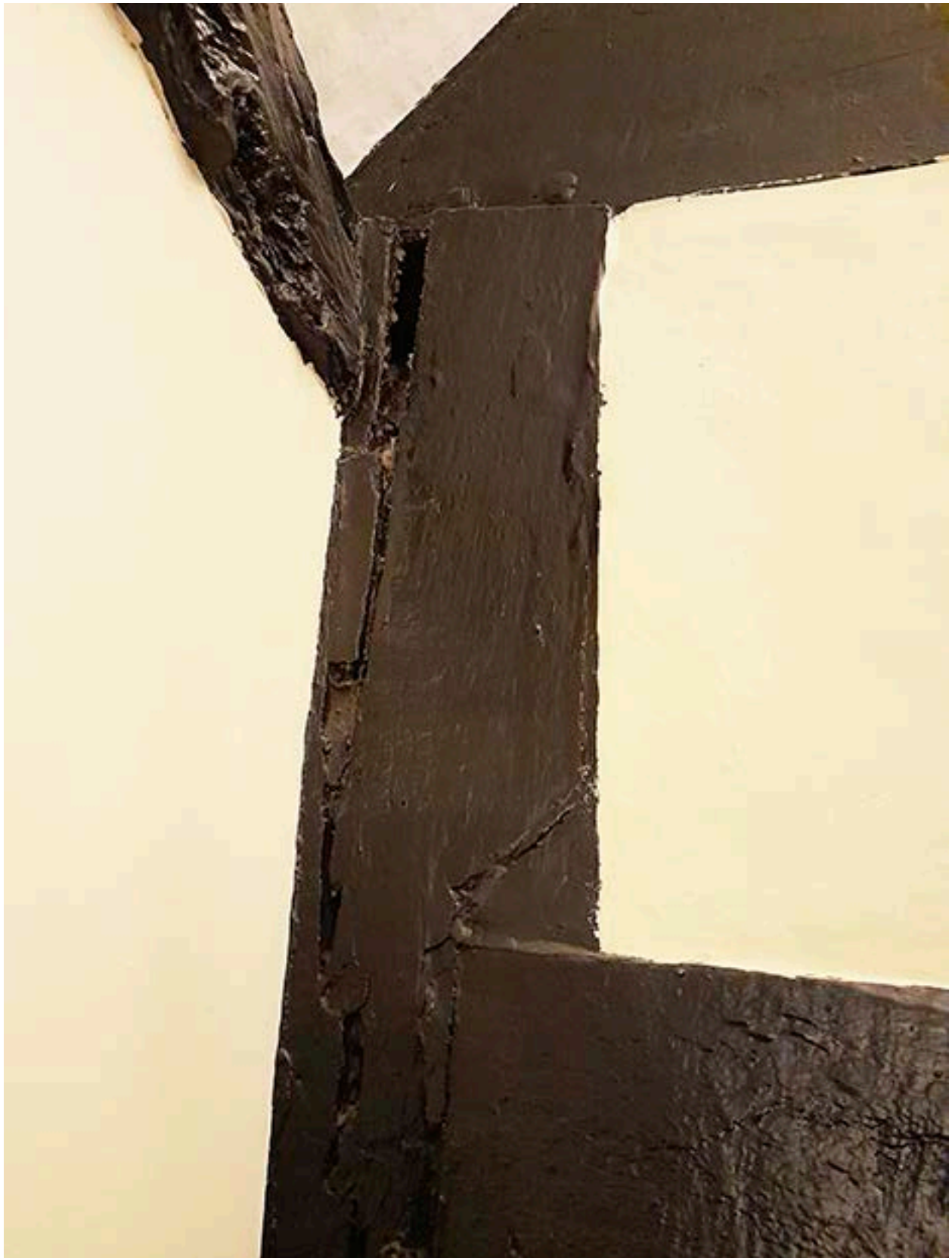
Figure 48: The southern wall post and wall plate (top left) in the fourth truss from the west. [Johanna Roethe © Historic England]
