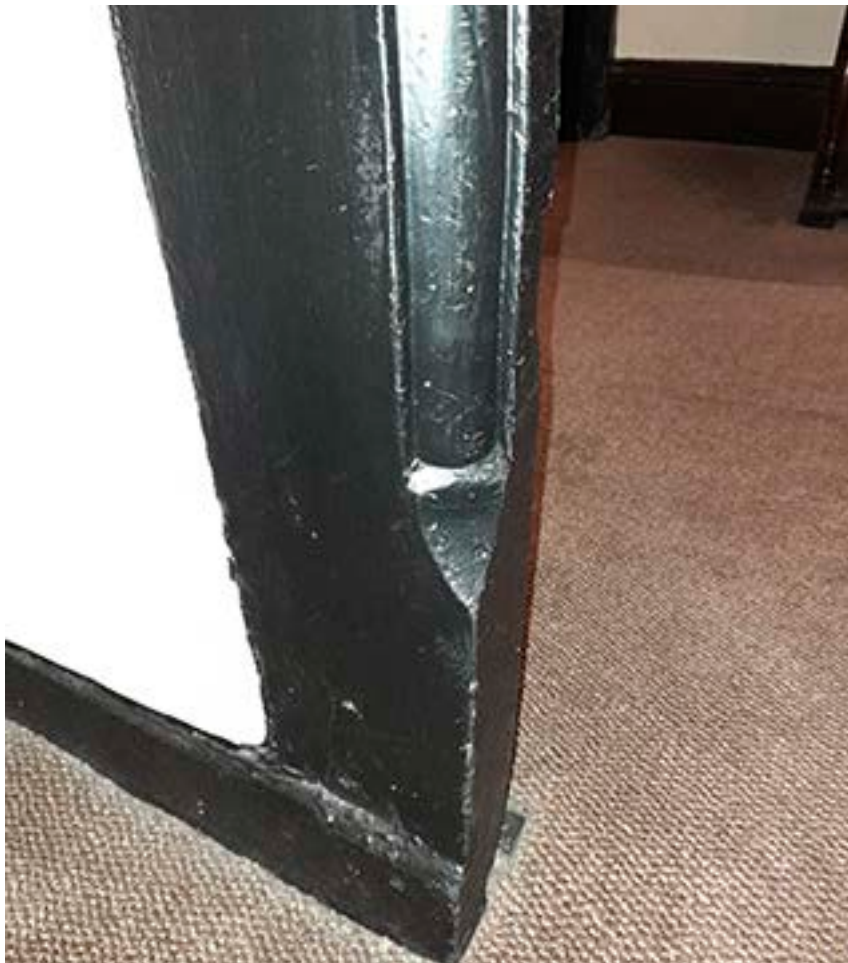
Figure 58: Detail of the ovolo-moulded door frame with scroll chamfer at first-floor level. [Johanna Roethe © Historic England]
