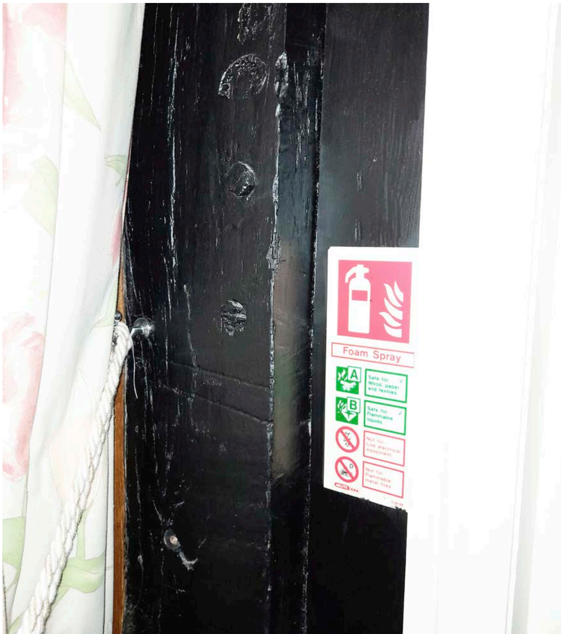
Figure 77: The redundant peg holes and possible carpenter’s mark in the third post from the east on the north wing’s south side, at first-floor level. [Johanna Roethe © Historic England]
