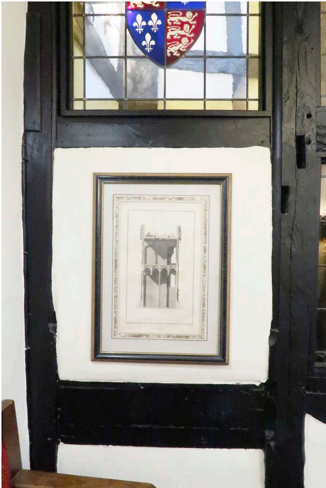
Figure 56: The lower part of the chamfered and stopped doorway on the first floor, with later infilling [Johanna Roethe © Historic England]
