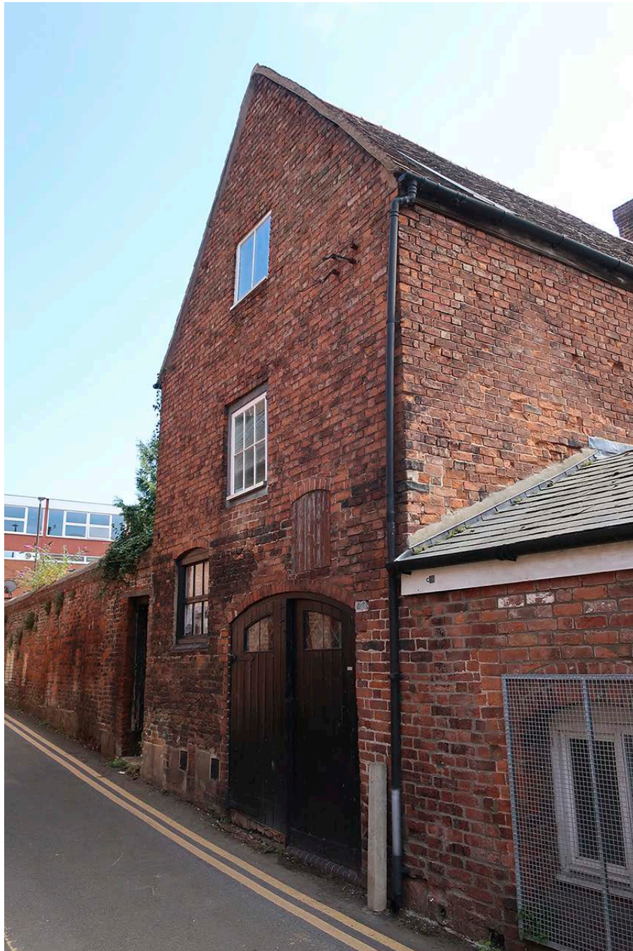
Figure 90: The north elevation of the stable block from Red Lane, seen from the north-west. [Johanna Roethe © Historic England]
