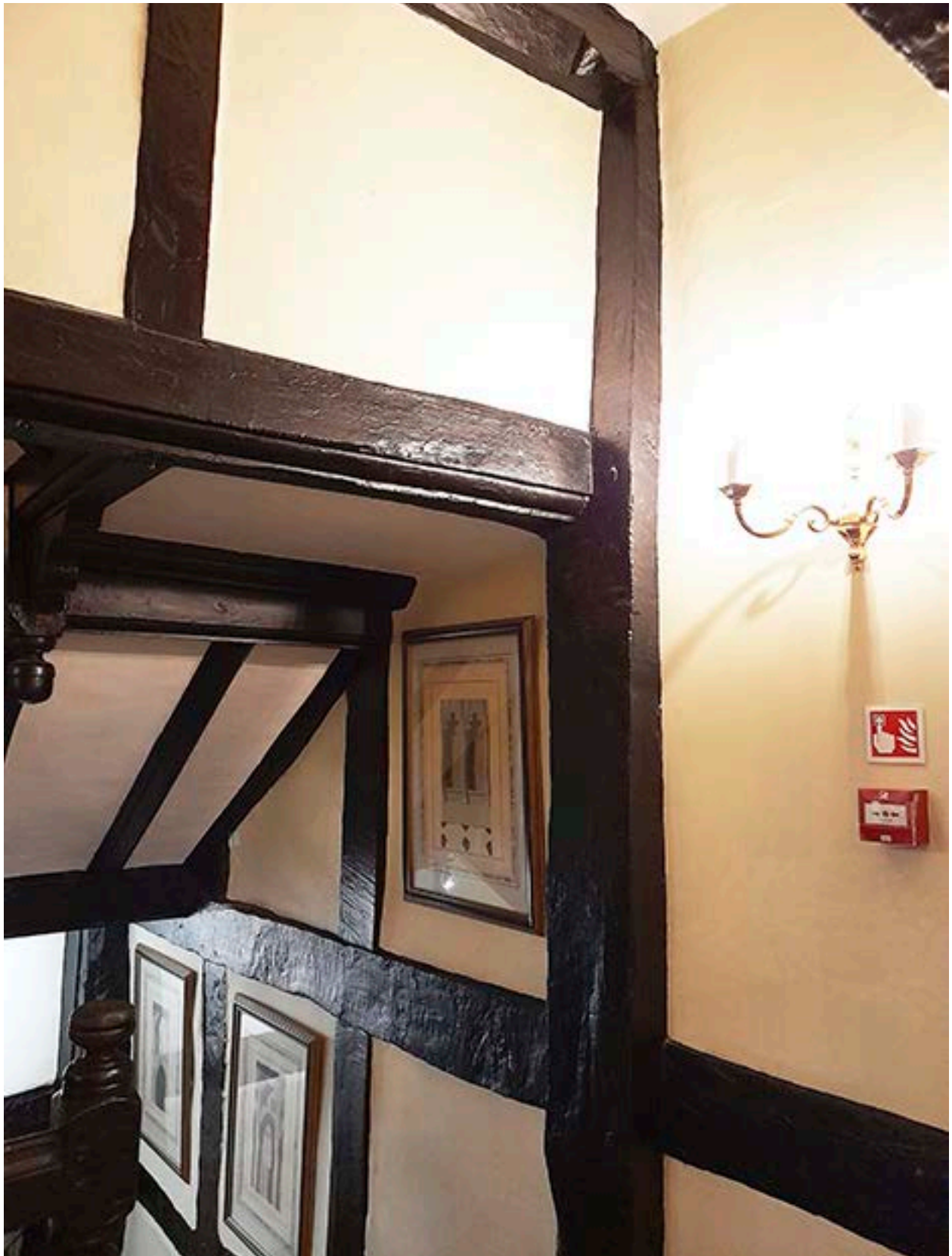
Figure 61: The ovolo-moulded trimmer at first-floor level. [Johanna Roethe © Historic England]
