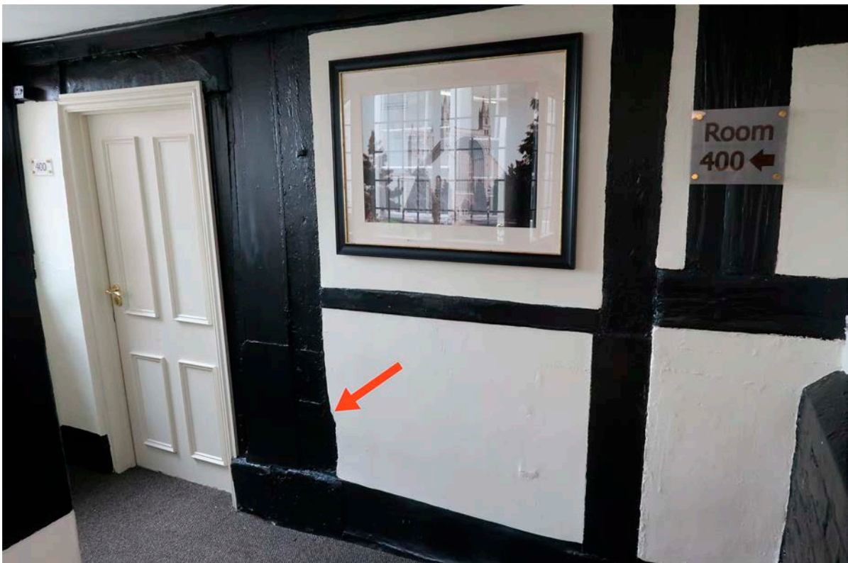
Figure 76: The location of the former doorway at the east end of the north wing's south elevation. The arrow indicates the potential chamfer stop. [Johanna Roethe © Historic England]
