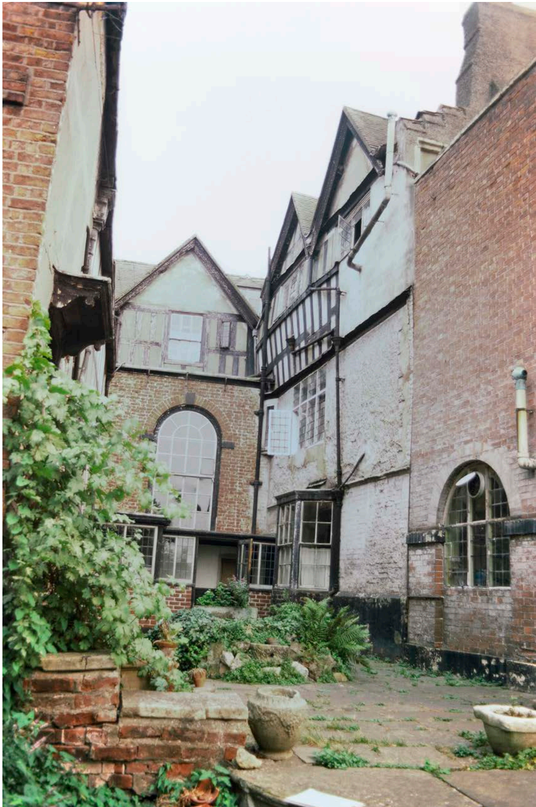
Figure 28: A photograph of the rear (west) elevation taken by Stanley Jones in about 1967-8. [© Historic England Archive, SJC01/03/0014]
