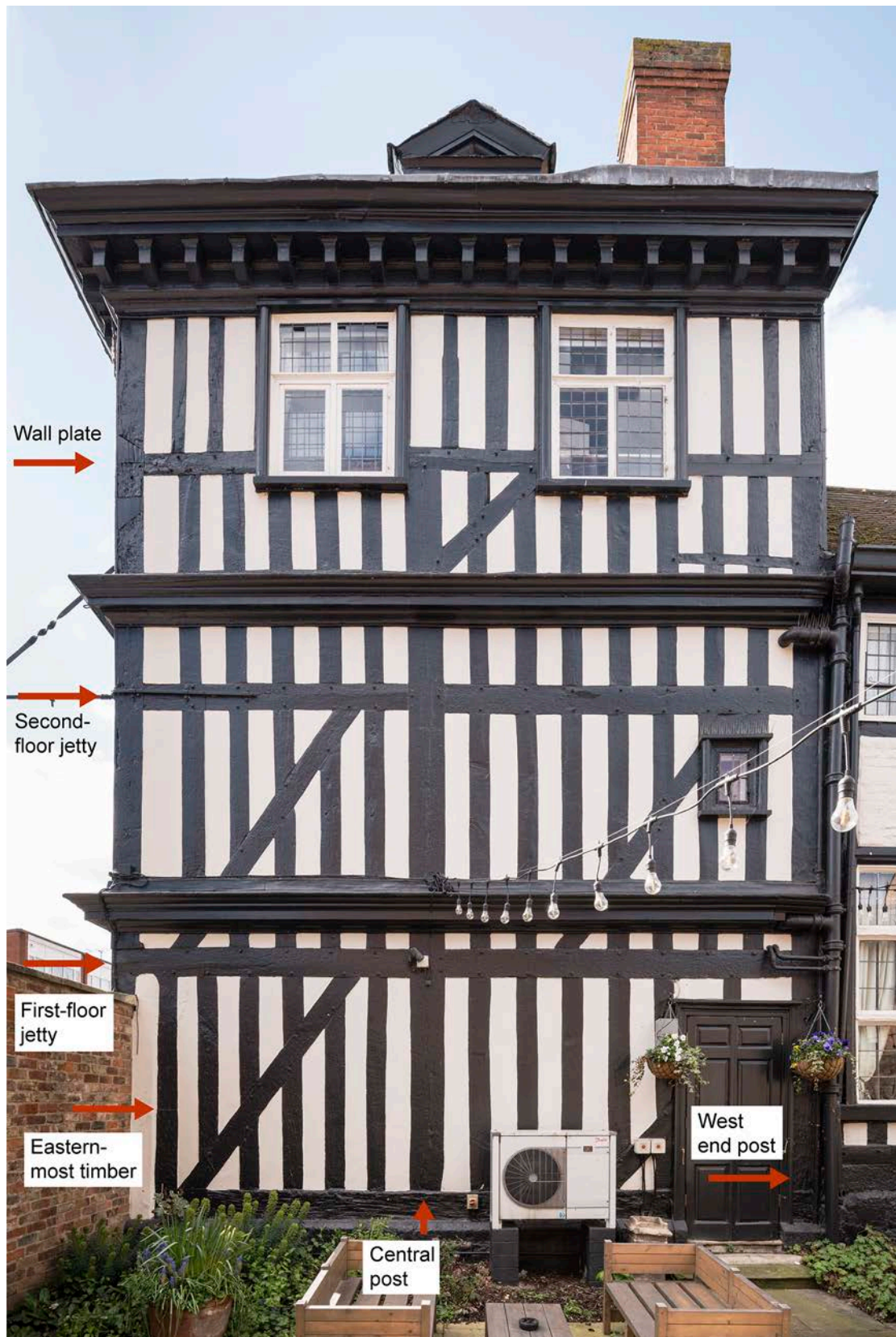
Figure 36: The north elevation of the front range, annotated with key original features. [Steven Baker © Historic England Archive, DP325759]
