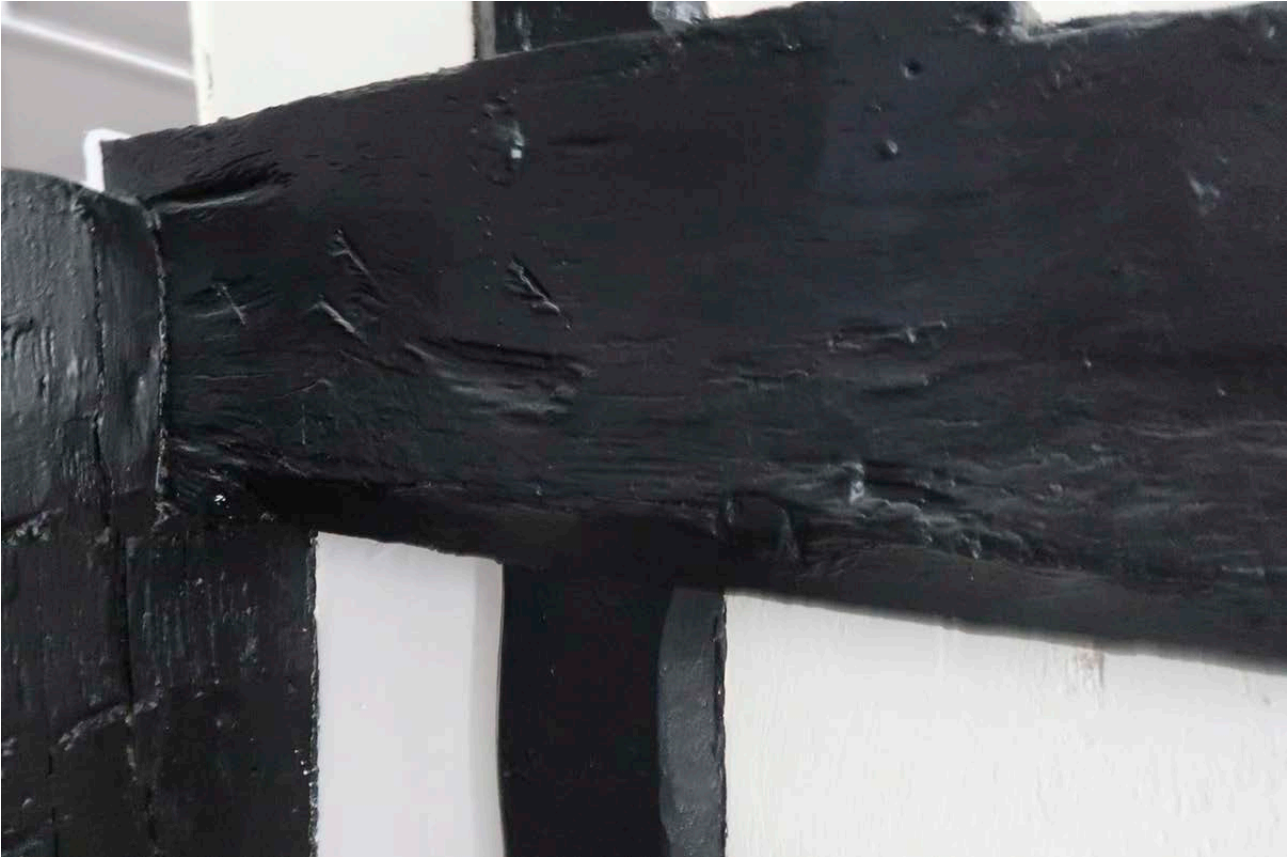
Figure 38: Chamfer, straight stop and peg hole on the underside of the wallplate at the north-east corner of the front range, indicating the possible location of an original window. [Johanna Roethe © Historic England]
