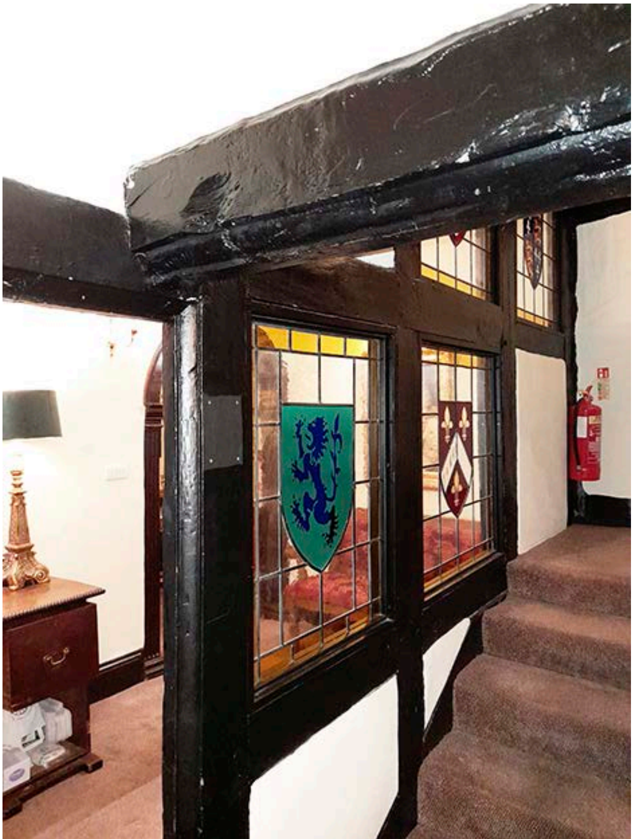
Figure 57: The north wall of the stairwell at first-floor level, with the blocked door to the half-landing at the far end. [Johanna Roethe © Historic England]
