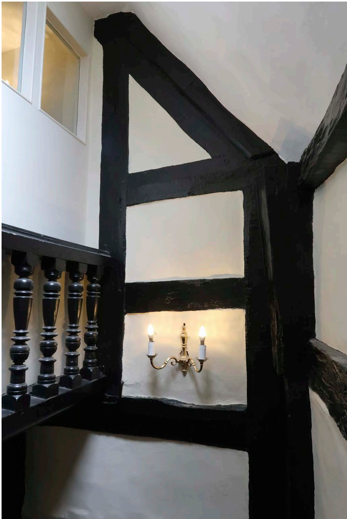
Figure 51: The south end of the easternmost truss of the south wing at attic level. [Johanna Roethe © Historic England]
