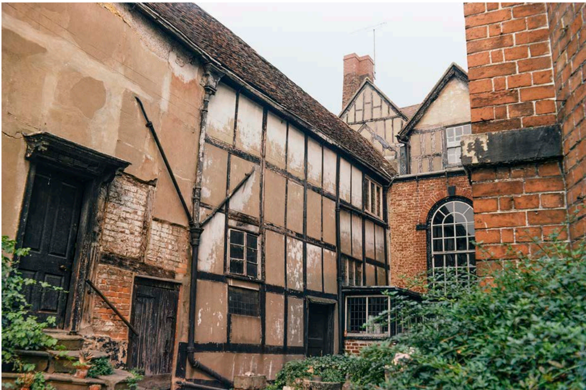
Figure 29: A photograph of the west elevation of the front range and the south elevation of the north wing (left) taken by Stanley Jones in about 1967-8. [© Historic England Archive, SJC01/03/0015]
