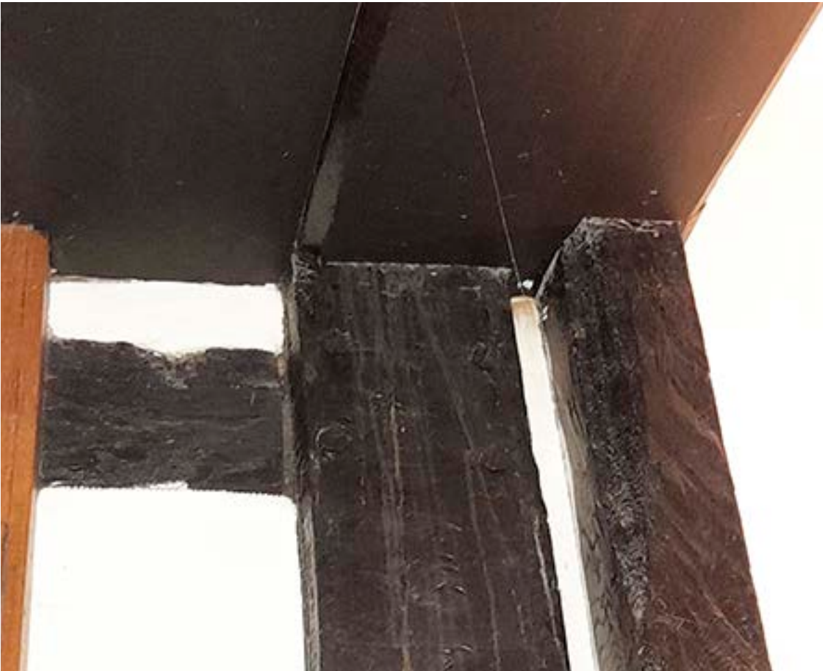
Figure 63: A wall post (centre) in the north wall of the south wing, at first-floor level, with the post relating to the stairwell enclosure to the right. Above is a boxed-in beam and to the left a later window frame. [Johanna Roethe © Historic England]
