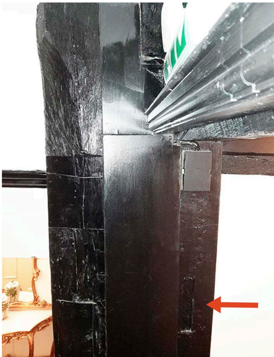
Figure 67: The junction of the front range's west elevation and the south-east corner of the north wing, seen at first-floor level. The north wing's south-east corner post is to the right, a modern timber at the centre, and a post belonging to the front range to the left. The arrow indicates the location of a mortice. [Johanna Roethe © Historic England]
