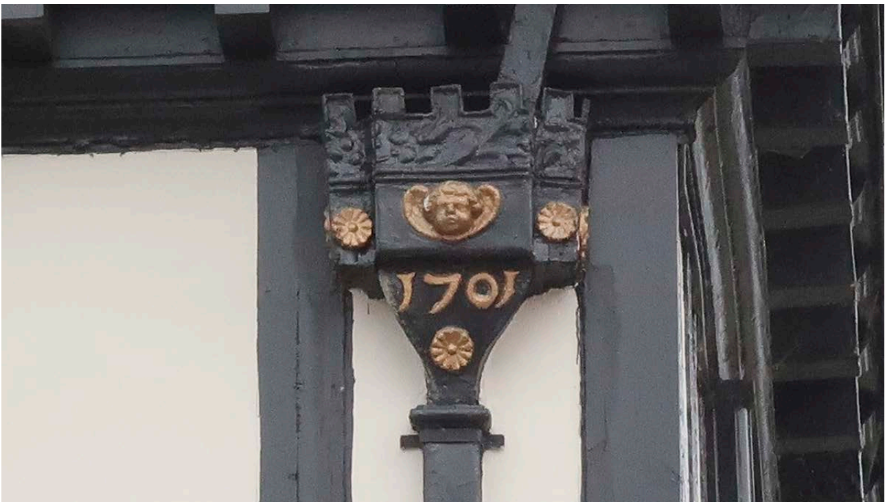
Figure 79: One of the 1701 rainwater hoppers. [Johanna Roethe © Historic England]
