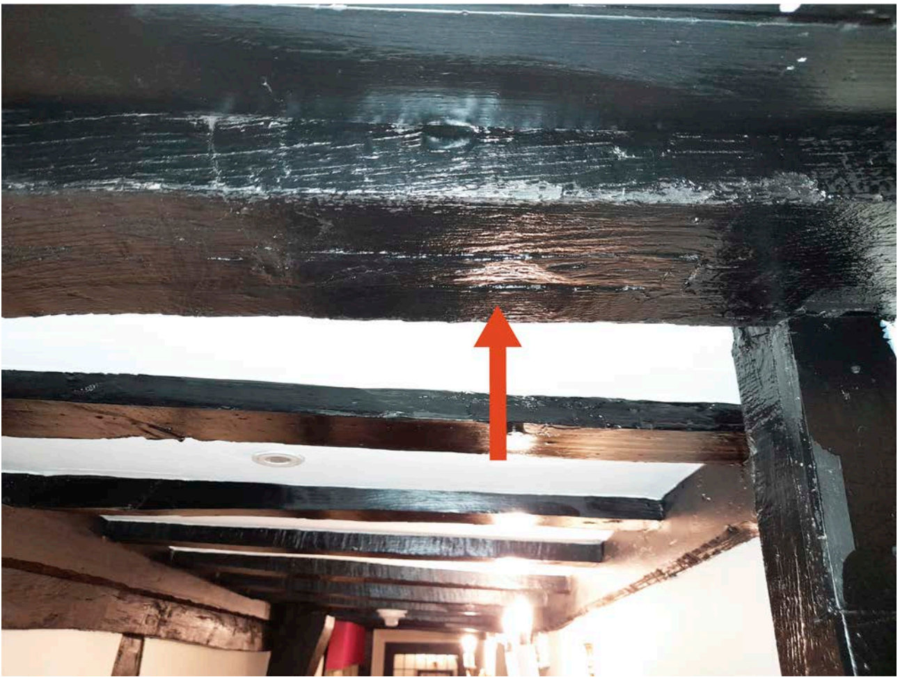
Figure 78: The modern post (left) in the location of the fourth post from the east in the north wing. The arrow indicates the empty mortise in the tie beam for a diagonal up-brace with two peg holes above. [Johanna Roethe © Historic England]
