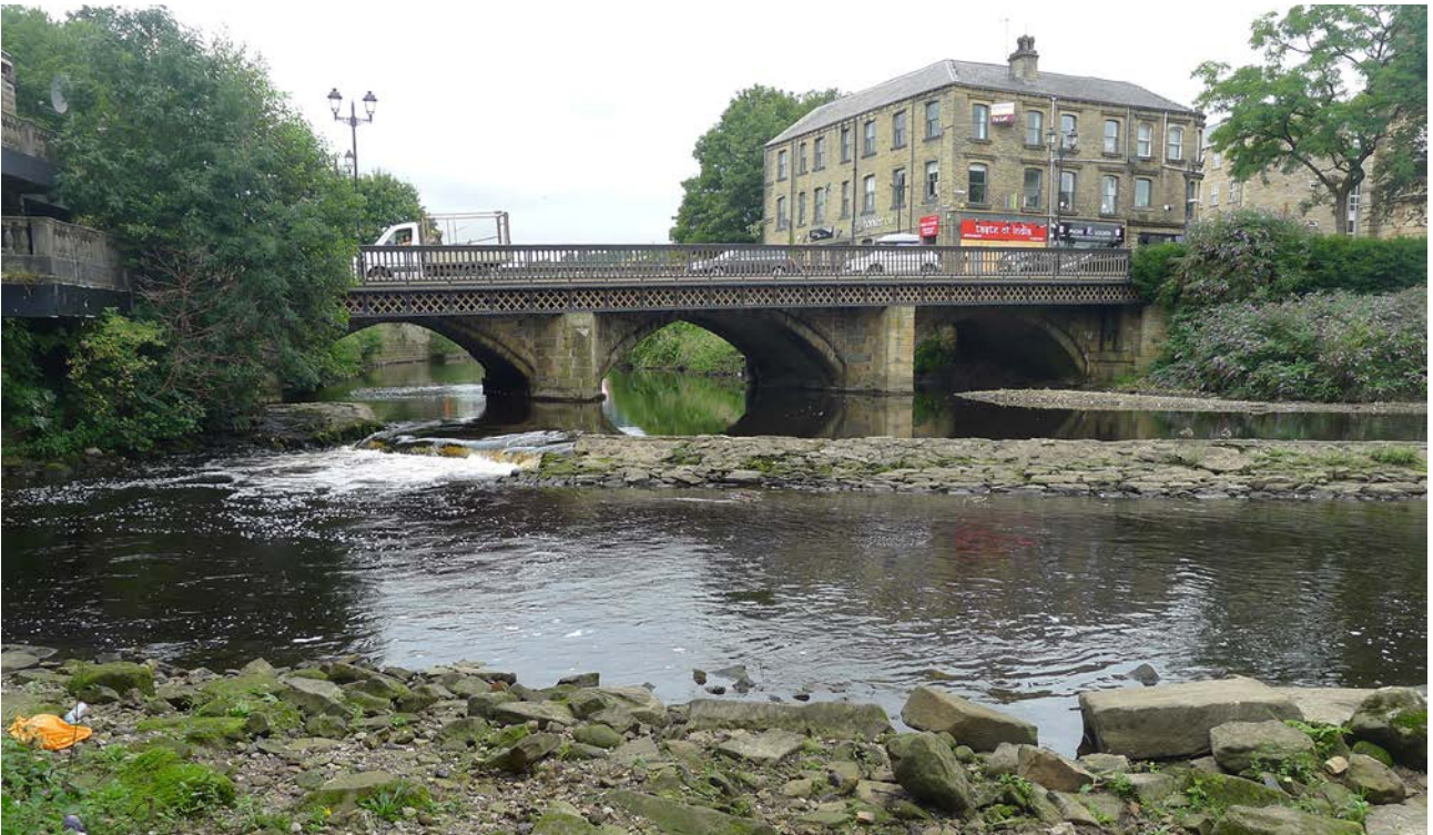
Figure 64: Eastern side of County Bridge showing the older stone bridge surmounted by the late 19th-century wider deck and iron balustrade, viewed from the south-east. [Lucy Jessop, 2021 © Historic England].
