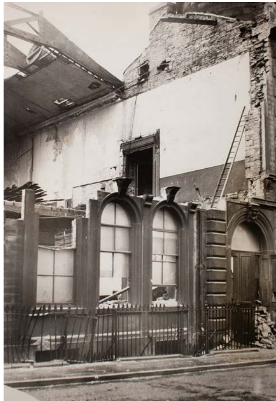
Figure 70: A photograph showing the demolition of the rear wing of the Town Hall, 1963. [Calderdale Libraries, 34 072 897 Courtesy of Halifax Courier].
