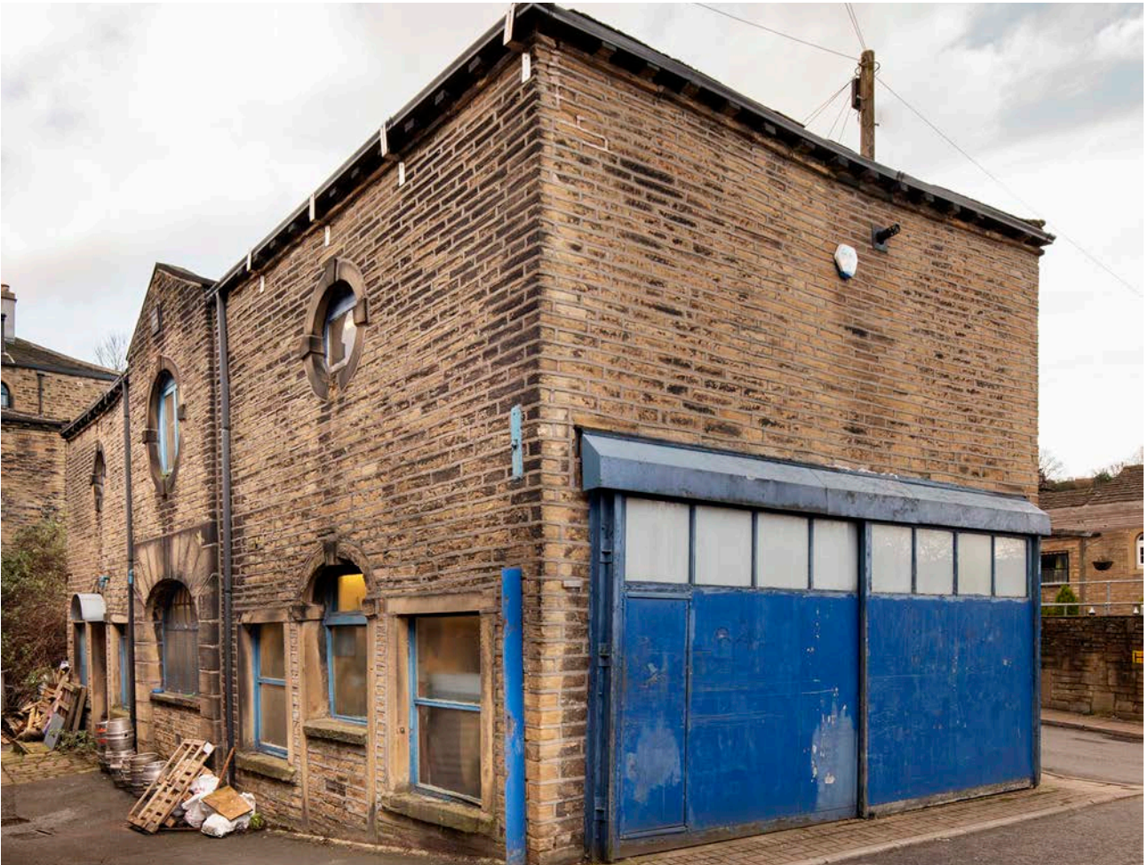
Figure 55: Former late 18th-century stable at the corner of Croft Street and Old Cawsey, viewed from the south. [James O. Davies, 2024 © Historic England, DP436986].
