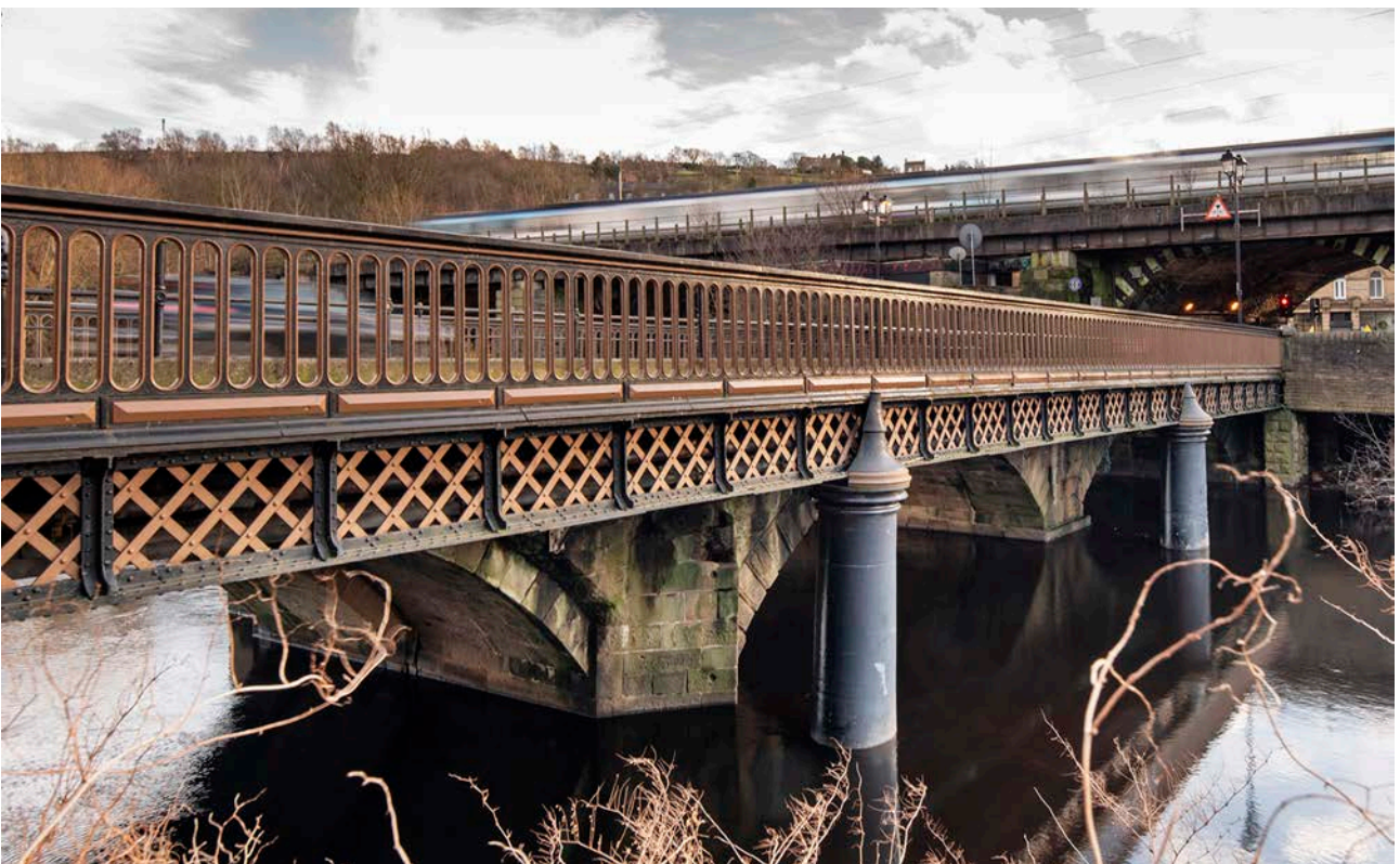
Figure 65: Western side of County Bridge showing the older stone bridge surmounted by the late 19th-century wider deck and iron balustrade, viewed from the north-west. [James O. Davies, 2024 © Historic England, DP437025].
