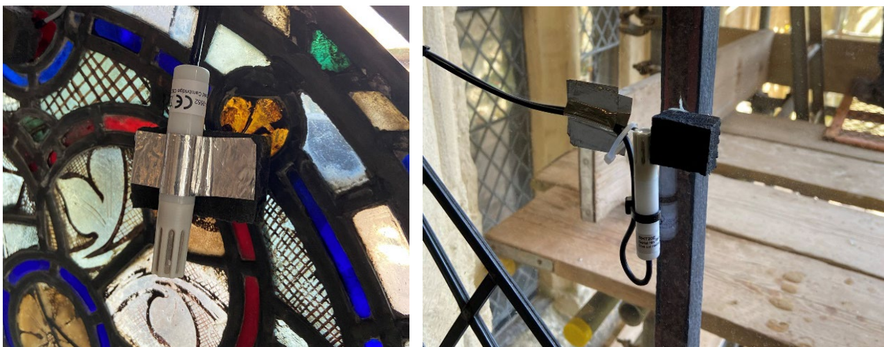
Figures 35 and 36: Relative humidity/ambient temperature and surface temperature sensors, attached to the stained glass (left) and modern glazing (right).
