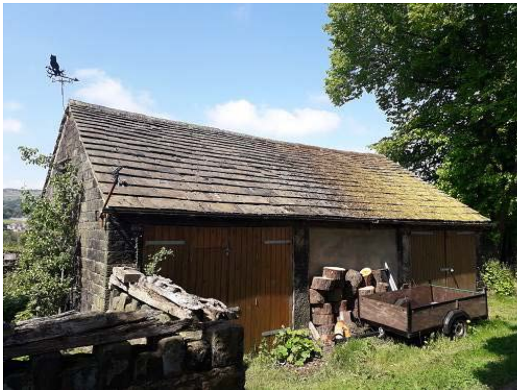
Figure 4c/d; Views of the open trusses to the west cross wing with truss 11 in the foreground (top) and the building to the driveway (bottom) (photographs Robert Howard)
