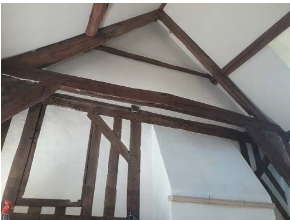
Figure 4a/b: Views of the open hall trusses, truss 7 (top), truss 8 (bottom) (photographs Robert Howard)
