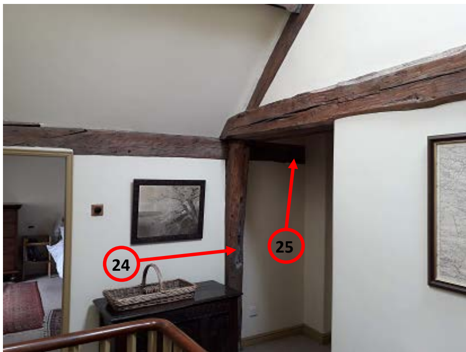
Figure 5c/d: Annotated photographs to help locate sampled timbers; open hall viewed looking east towards truss 6 (top), and east cross-wing, truss 2, viewed from the south (bottom) (photographs Robert Howard)
