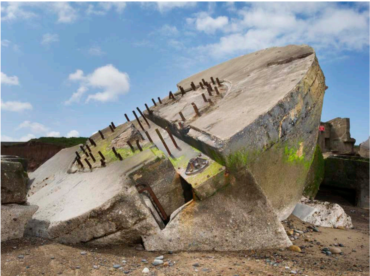
Figure 2: A WWI gun emplacement at Kilnsea, East Yorkshire has collapsed onto the beach due to coastal erosion. © Historic England Archive
