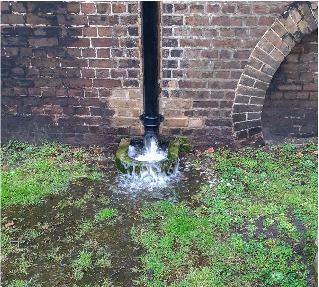
Figure 5: Rainwater systems can be overwhelmed during heavy downpours and adaptation measures may be required to increase capacity. See Appendix I, Case Study 4.
