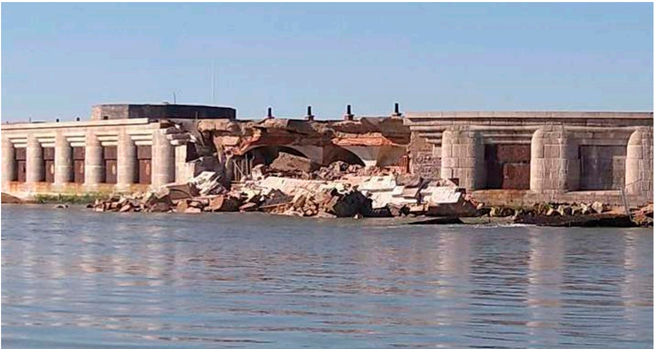
Figure 11: The collapsed section of Hurst Castle's C19 East Wing in 2021. © World Monuments Fund Britain
