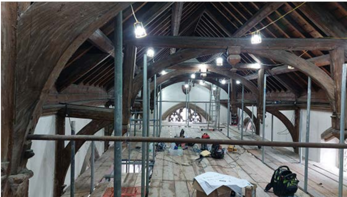
Figure 3a/b: General views of the Chapel roof viewed looking east to west (top) and west to east (bottom) [photographs Robert Howard]
