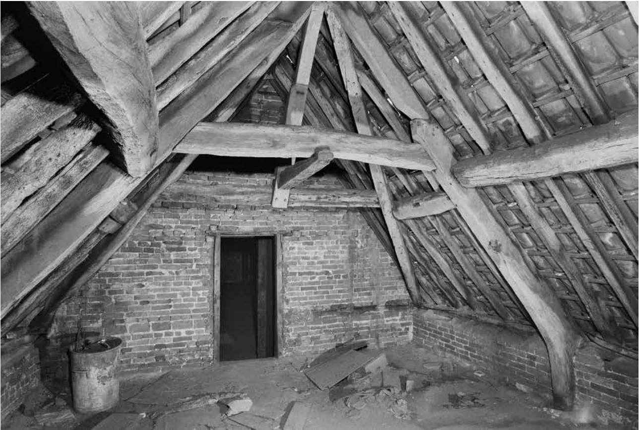
Figure 33: Rear range to the Clinton Arms prior to demolition in the 1980s. The upper cruck roof may have been retained in the subsequent redevelopment. [© HEA AA107262.]
