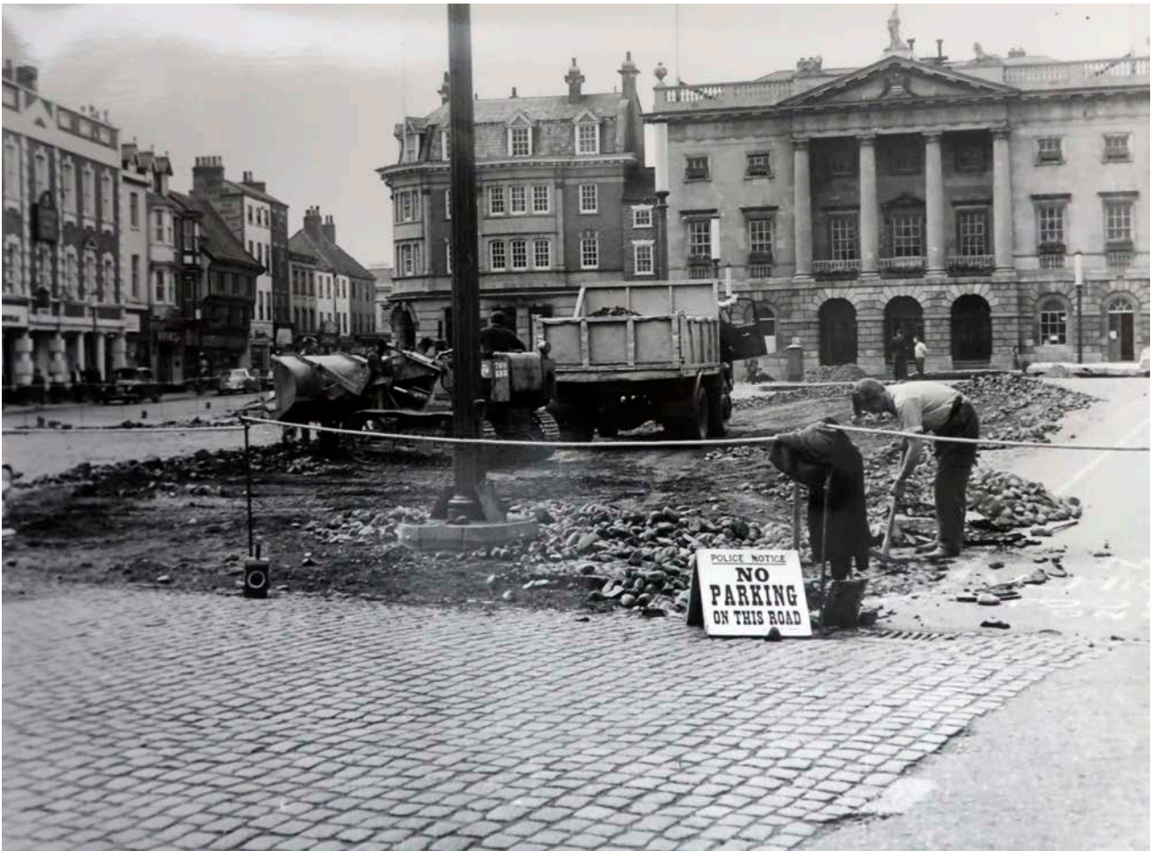
Figure 22: Relaying of the cobbles from the centre of Market Place in 1965. [© Newark Resource Centre (no reference number).]
