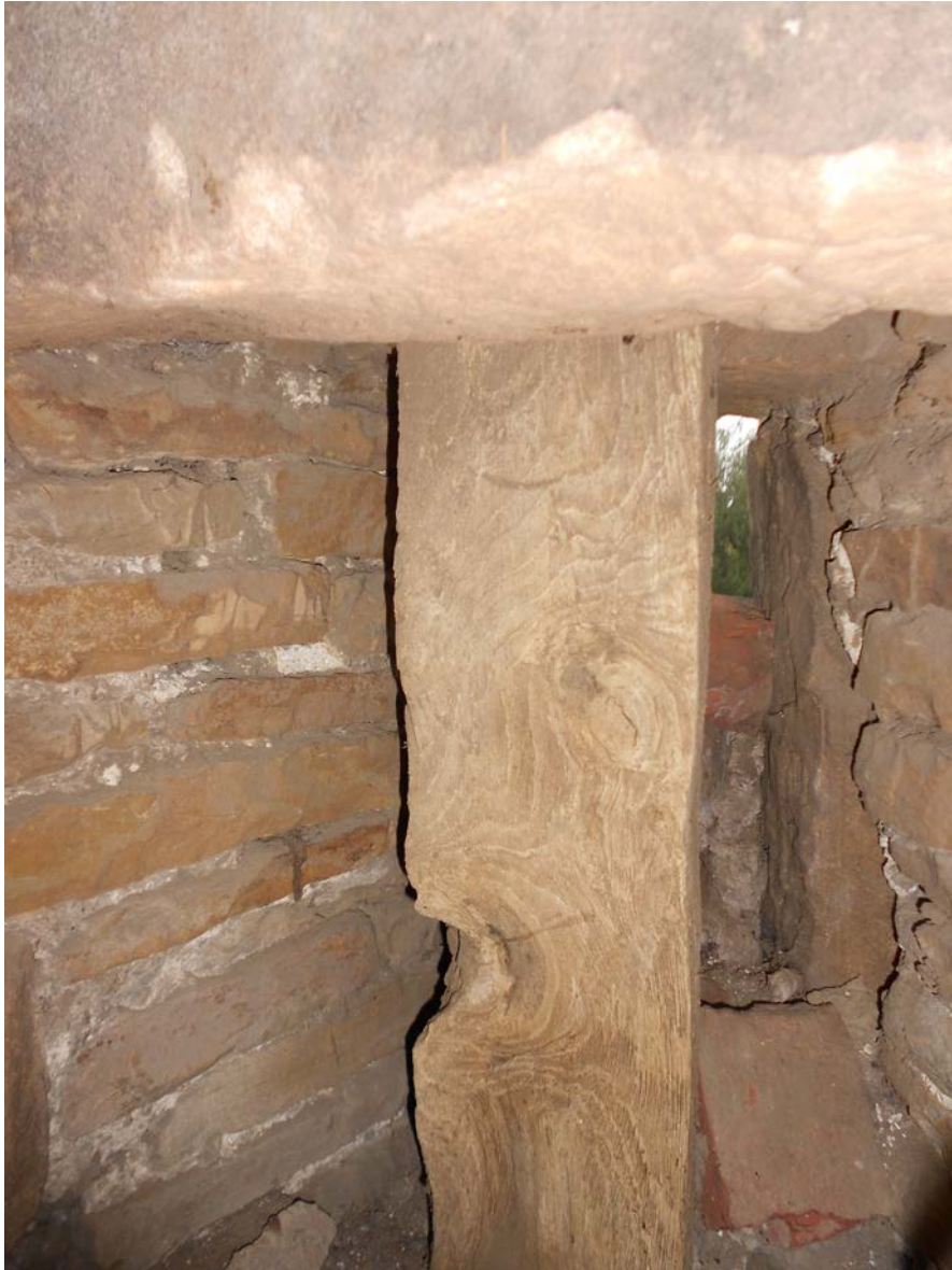
Figure 4: Timber within a window reveal, thought to be part of the original framing of the cruck barn (photograph by Martin Bridge)
