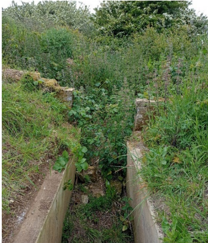
Figure 13: View looking west into collapsed shelter, D2 HAA battery, 31st May 2023.
