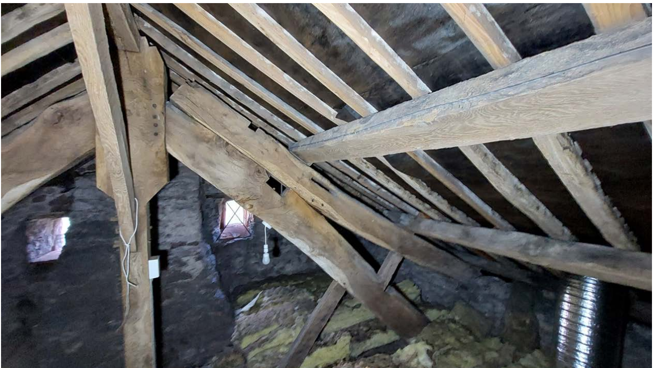
Figure 10: Roof, secondary rafters of truss 1, photograph taken from the south. [Alison Arnold]
