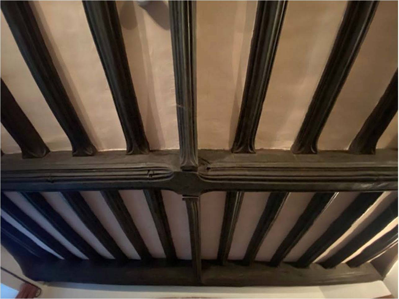
Figure 7: Ceiling/floor frame in the hall, photograph taken from the north. [Alison Arnold]
