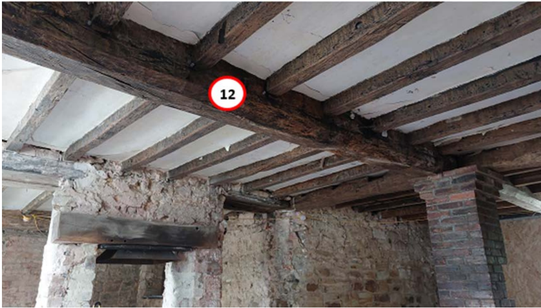
Figure 3e: North Cottage, south bay, viewed looking north east. [photograph Robert Howard]
