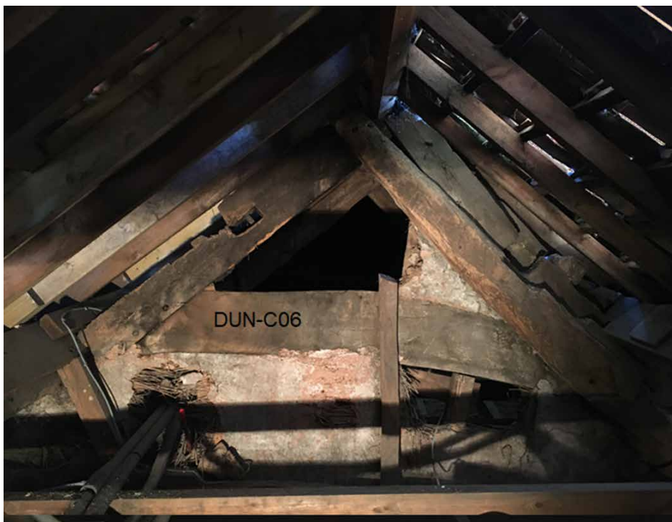
Figure 6: T4 is a jointed cruck truss. Sampled timber marked DUN-C06, photograph taken from the north. [Alison Arnold]
