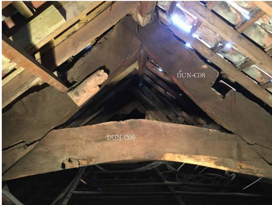
Figure 5: T3 is a jointed cruck. Sampled timbers marked DUN-C08 and DUN-C09, photograph taken from the north. [Alison Arnold]
