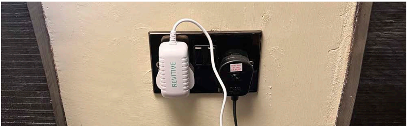
Figure 19: Electrical sockets © The Environmental Design Studio
