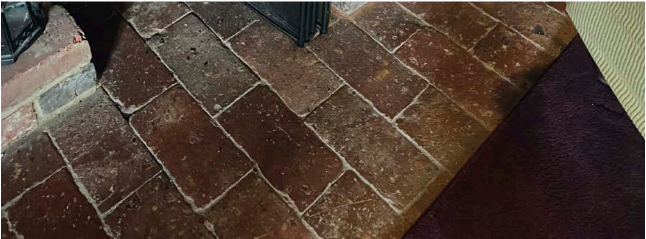
Figure 18: Living room floor © The Environmental Design Studio
