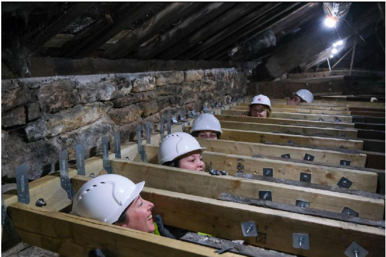
Figure 30 – Participants learning and doing on site Participants conducting ceiling joist repairs to the church where their Summer School is hosted Historic England © All Rights Reserved
